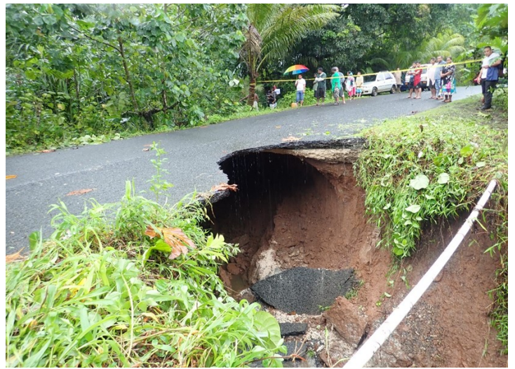
Damaged roads at Pohnpei
