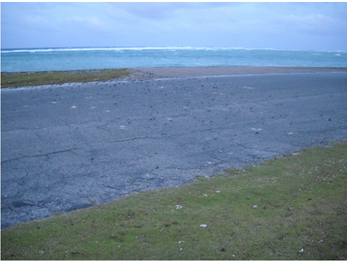
Picture. 1: Tides and Inundation pictures in Kwajalein (Pictures attached are day after evening high tide 4 Feb). The site is located north of runway on Roi Namur, near 9 24' 4.75"N, 167 28' 30.96E. Event is associated with northerly swell from northern Pacific storm. (Photo Credit: Mr. Eugene Bell, Kwajalein Atoll, RMI).
