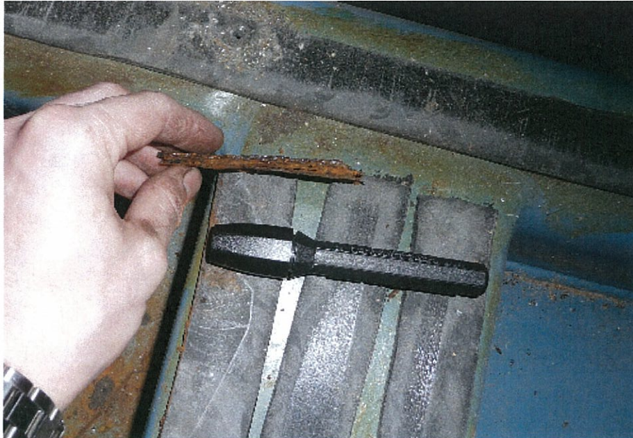
Figure 6: A piece of rust taken from the backing plate
