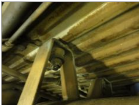
Figure 89 Image of corroded bolts of underframe equipment
