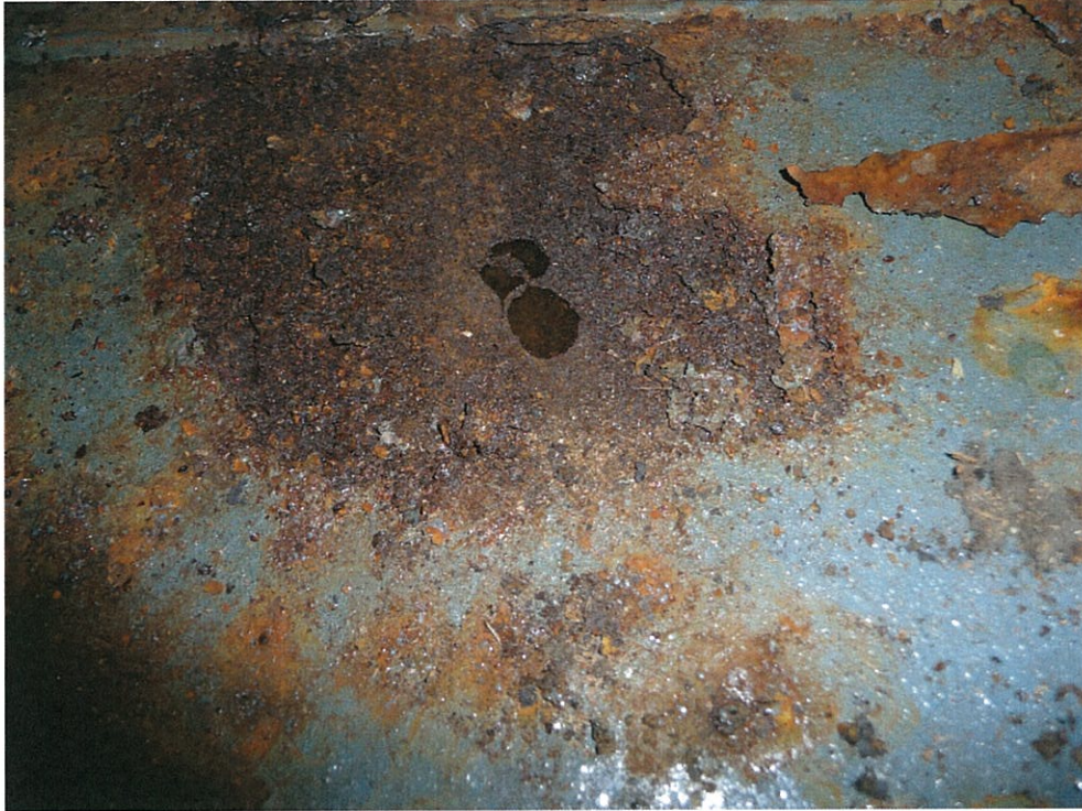
Figure 2: Area of corrosion on the headstock floor on EMU 23
