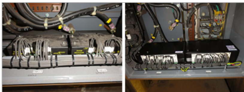
Figure 72 Image of door control unit
