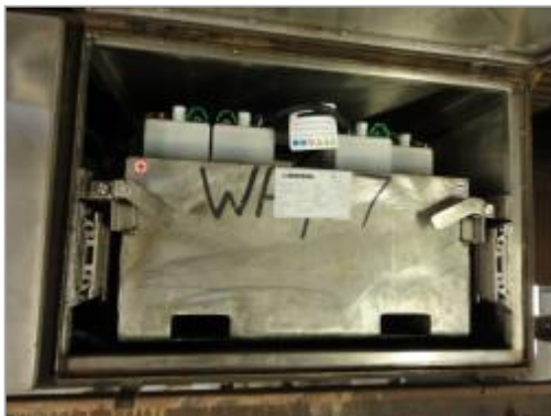
Figure 69 Image of battery bay
