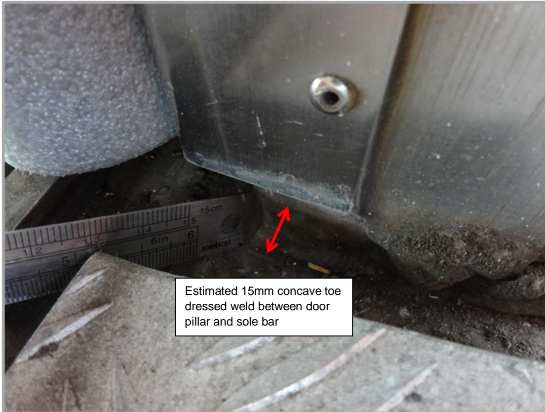
Figure 24 Railcar 236 welded joint between door pillar and solebar
