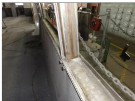
Figure 86 Image of corrosion residue on carbody structure after aluminium window frames are removed
