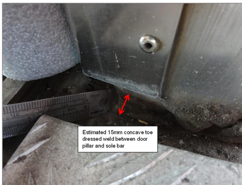
Figure 24 Railcar 236 welded joint between door pillar and solebar
