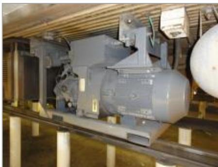
Figure 54 Image of main compressor of brake system
