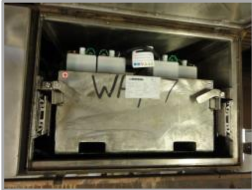
Figure 69: Image of battery bay
