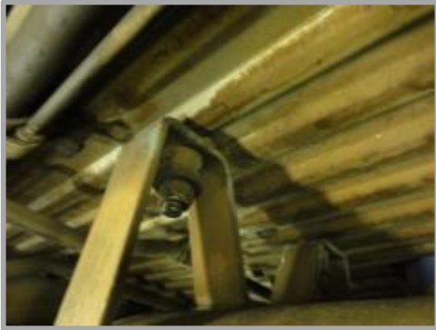
Figure 89: Image of corroded bolts of underframe equipment
