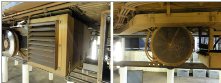
Figure 57 Image of brake resistor and fan
