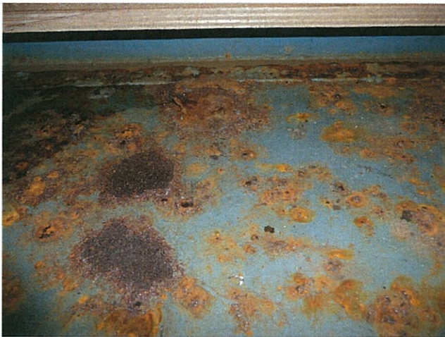
Figure 1a: Headstock Floor on EMU 23 showing corroded areas
