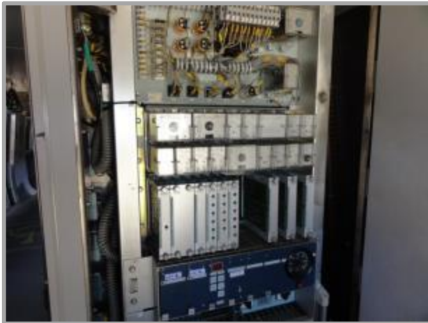
Figure 97: Image of relay box within drivers cab (unit 36)
