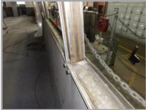
Figure 86: Image of corrosion residue on carbody structure after aluminium window frames are removed
