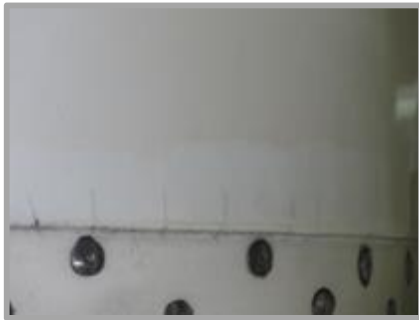
Figure 92: Image of fibreglass fatigue cracks
