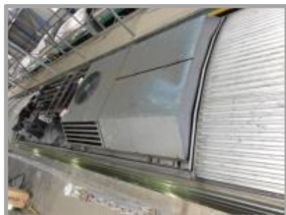
Figure 74: Image of HVAC unit
