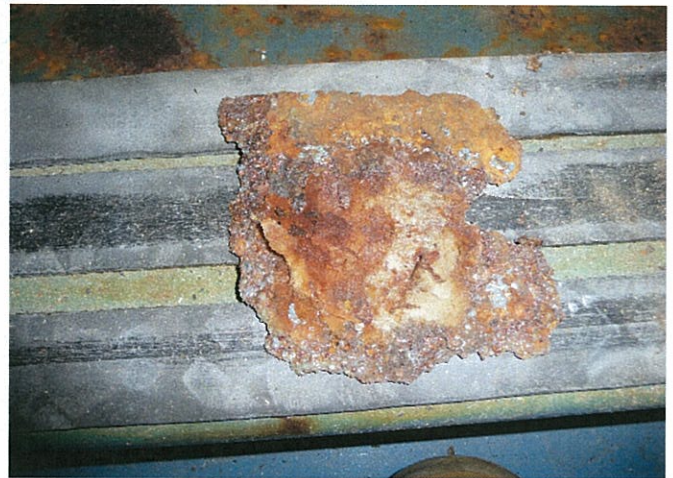
Figure 1b: A piece of rust that was taken from the headstock floor. (Note beam underneath is 100mm wide)
