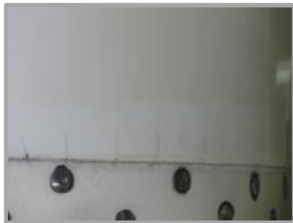
Figure 92: Image of fibreglass fatigue cracks
