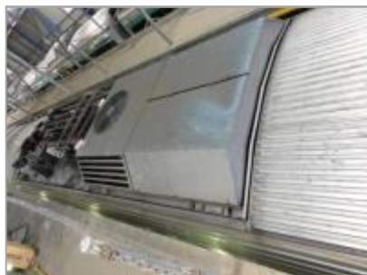
Figure 74 Image of HVAC unit
