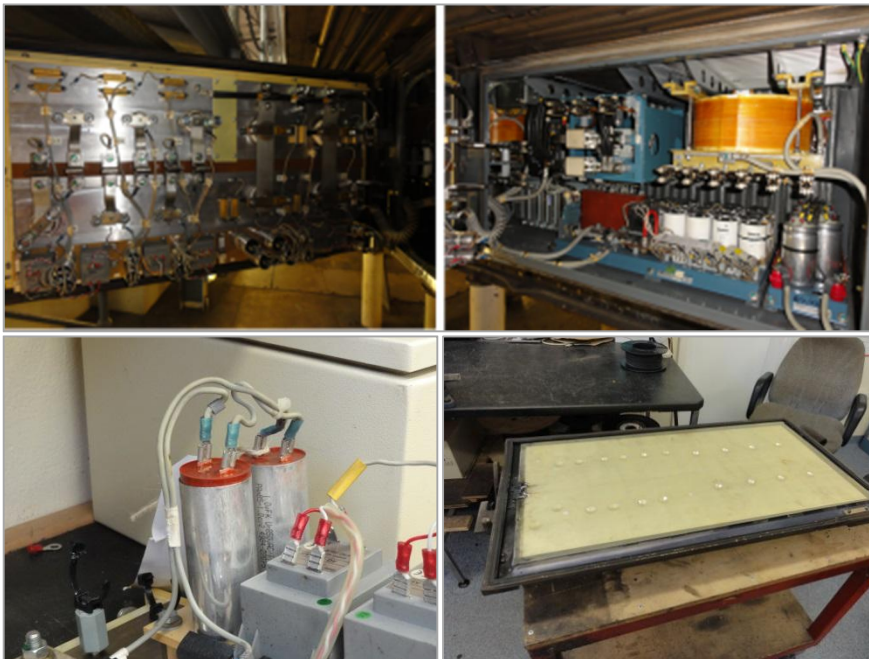
Figure 67 Image of auxiliary converter, capacitors and contactor, leaking capacitor, damaged plastic backing
