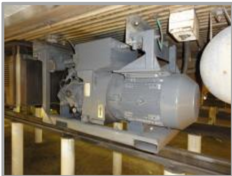
Figure 54: Image of main compressor of brake system
