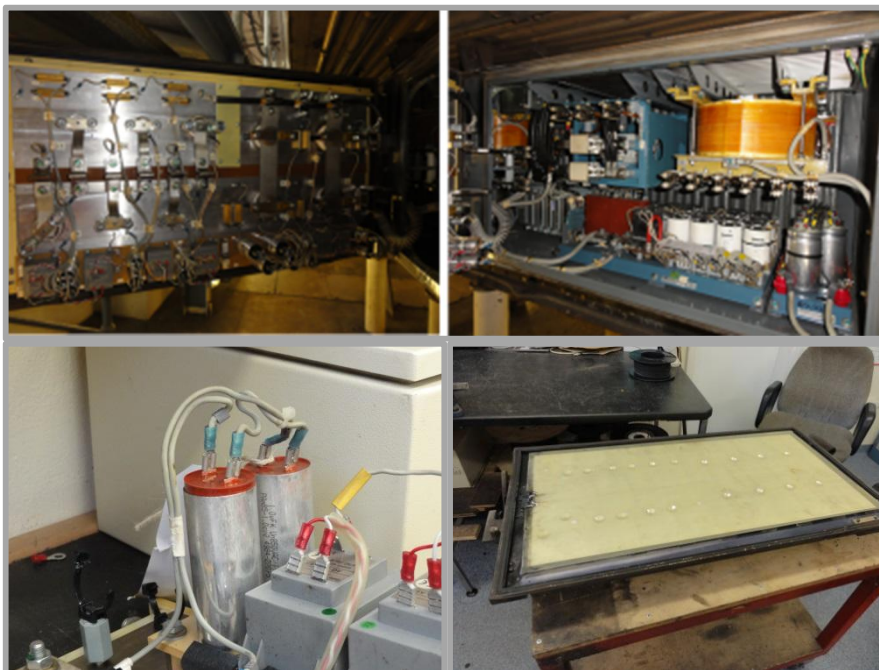
Figure 67: Image of auxiliary converter, capacitors and contactor, leaking capacitor, damaged plastic backing
