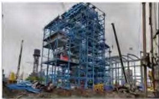
Power Plant II
