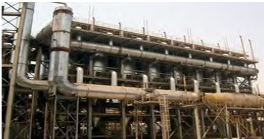
Figure 4.6 : Photograph of a Typical Bag Filter for Cleaning Crude BF Gas
