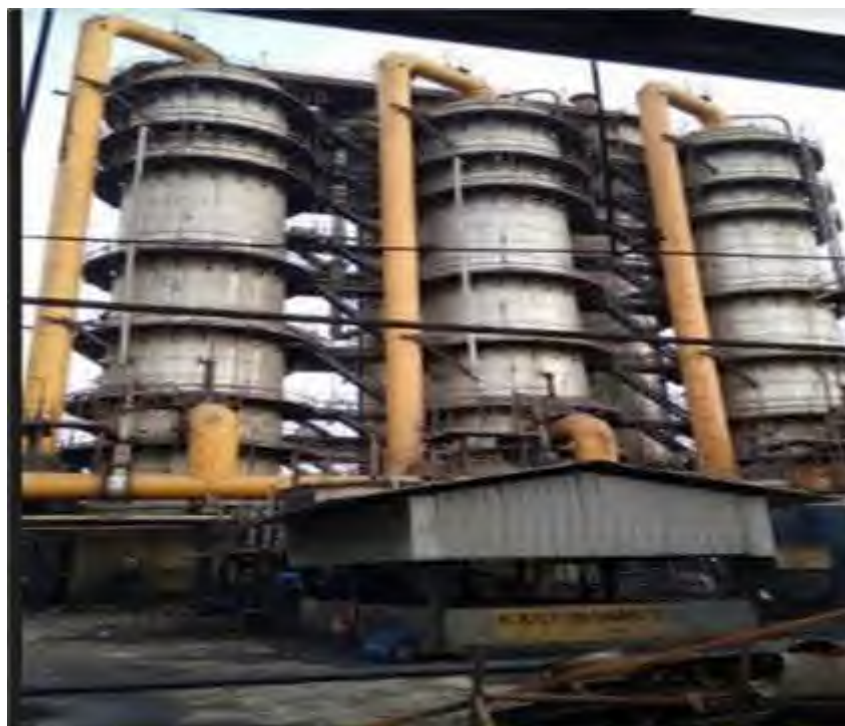
Figure 4.5 : Coke Oven Gas Desulphurization Plant
