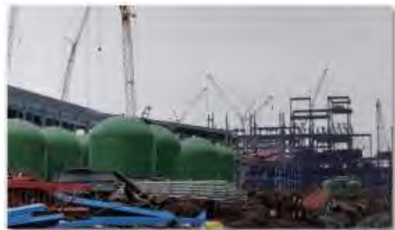
Filtration Unit of Blast Furnace II
