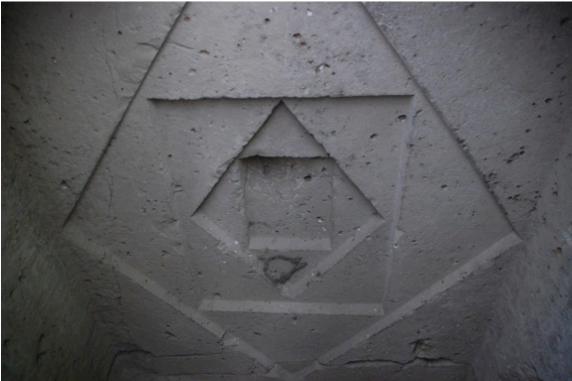
Figure 86: Emulation of a "lantern-roof" in the Gerdek Boğazı tomb at Karakoyunlu (Image source: Author)
