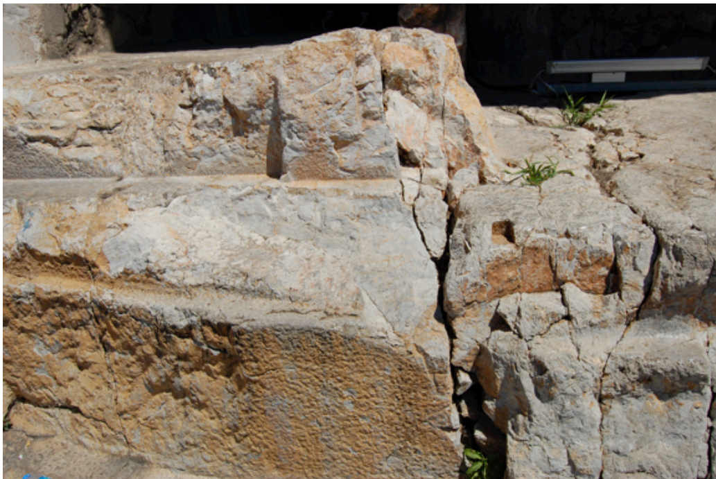
Figure 104: Discrepancy in foundation levels between Tombs B (right) and C (left) (Image source: Author)
