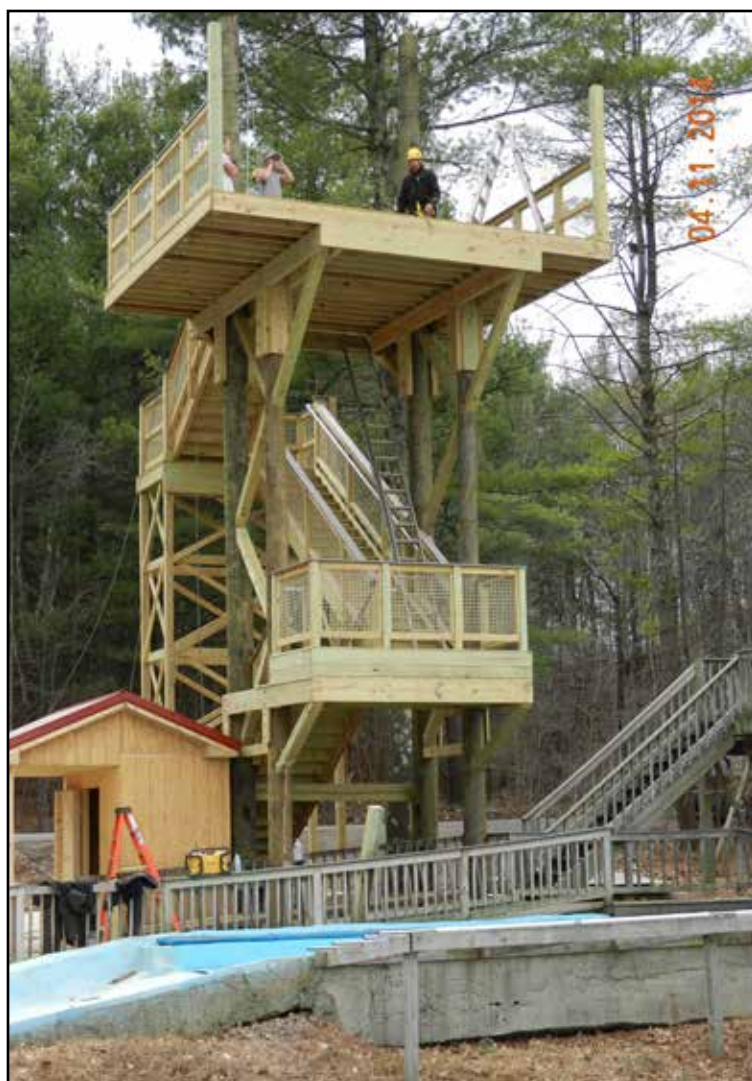
Construction is in the final phases on the Gravity Gorge Zipline tower, new this summer at Zoom Flume.
