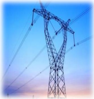
Two Independent Off-site Power Supplies
