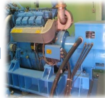
SBO Diesel Generators/ DEC Batteries
