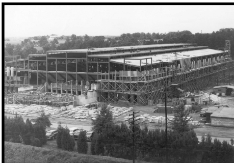
Construction began on Reynolds Coliseum in 1943, but was delayed many times during World War II.
