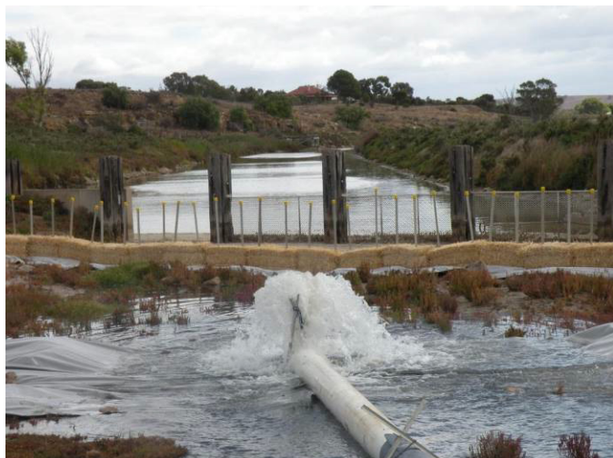
First day of emergency pumping at Rocky Gully Wetland, South Australia. March 31 st 2009.
