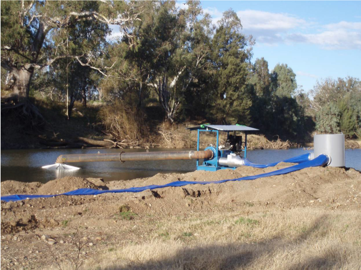
Figure 2: Experimental pumping station being tested during the pilot trial.
