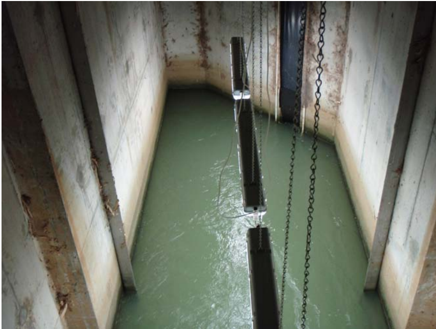
Figure 3: Artificial lighting suspended from the fishway grid mesh at Lock 8
