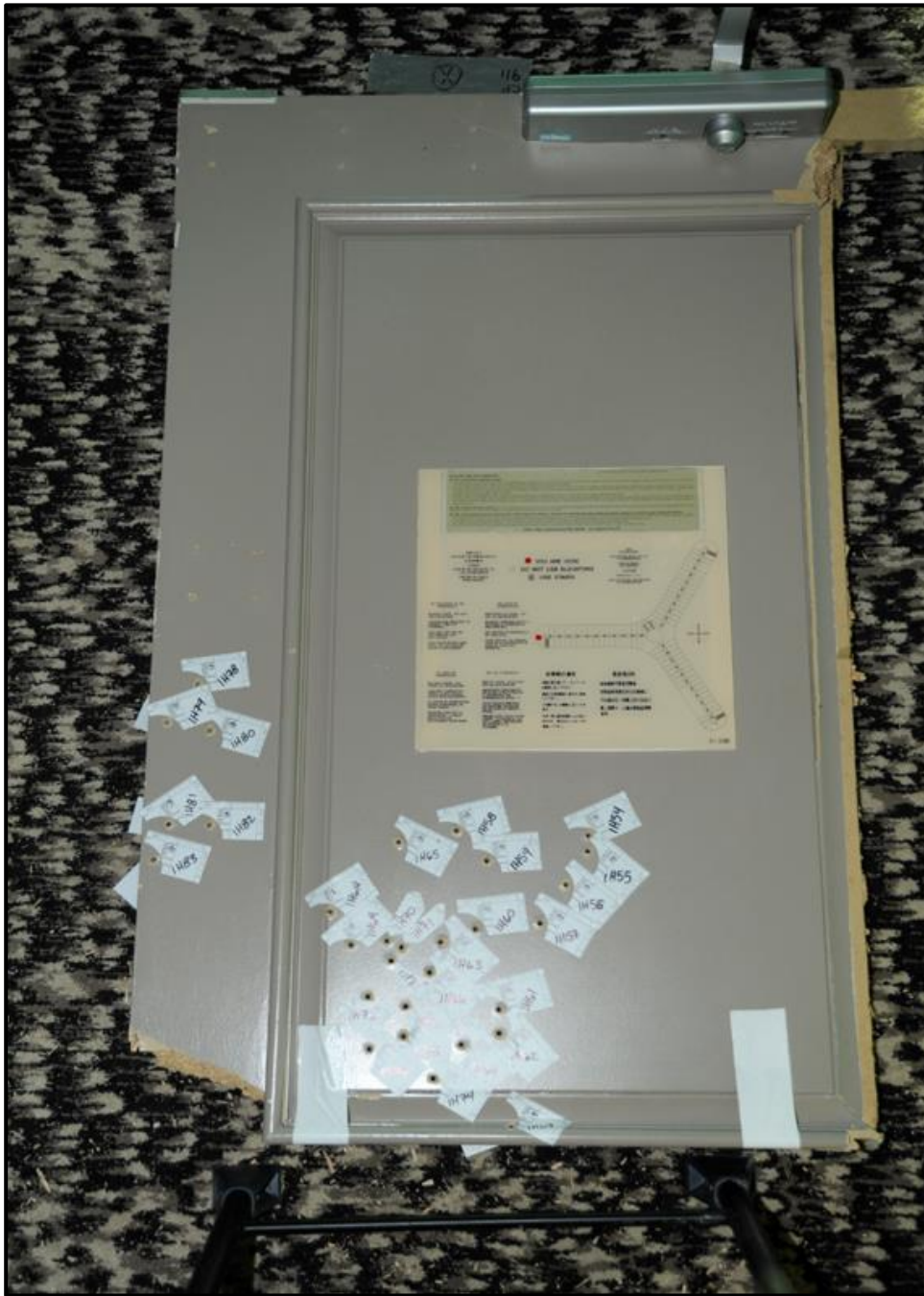
(Damage to entry door of room 32-135)
