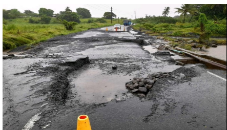
Figure 18: Rabulu road (Tavua) damaged due to continuous flooding on 17 th February, 2023. Source: fijivillage.
