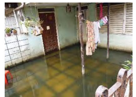
Flooded Area on West Side of the Station
