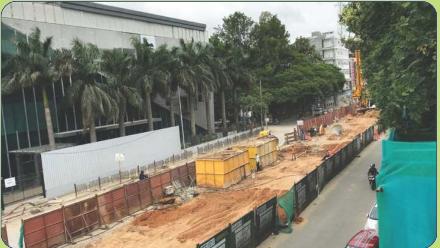
The Well-known Jayadeva Flyover demolition work was successfully completed by BMRCL as part of Phase-2 Project Work
