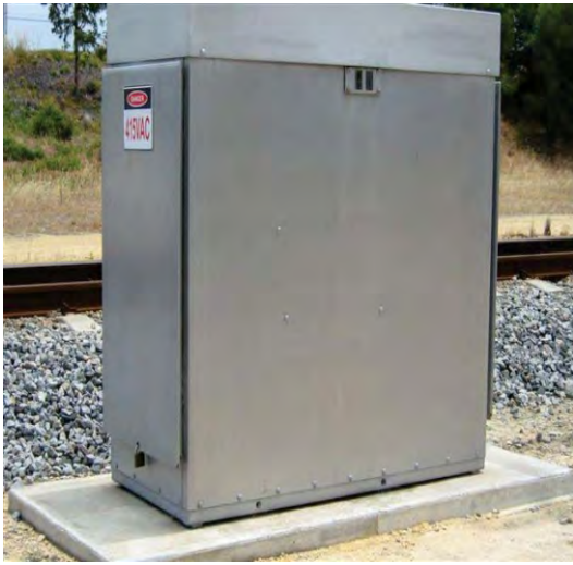
EST Electrical Supply Transformer
