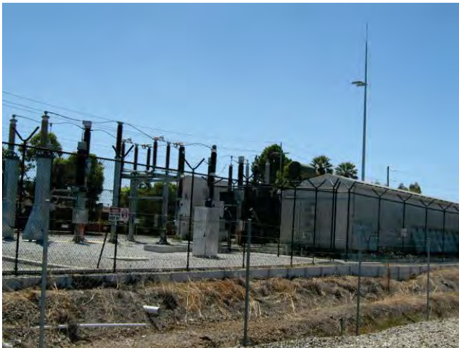
SFS Sub Feeder Station
