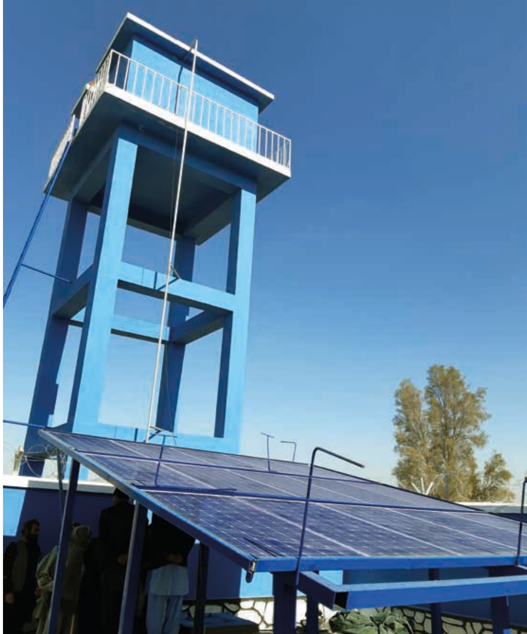
Solar powered water system in Afghanistan
