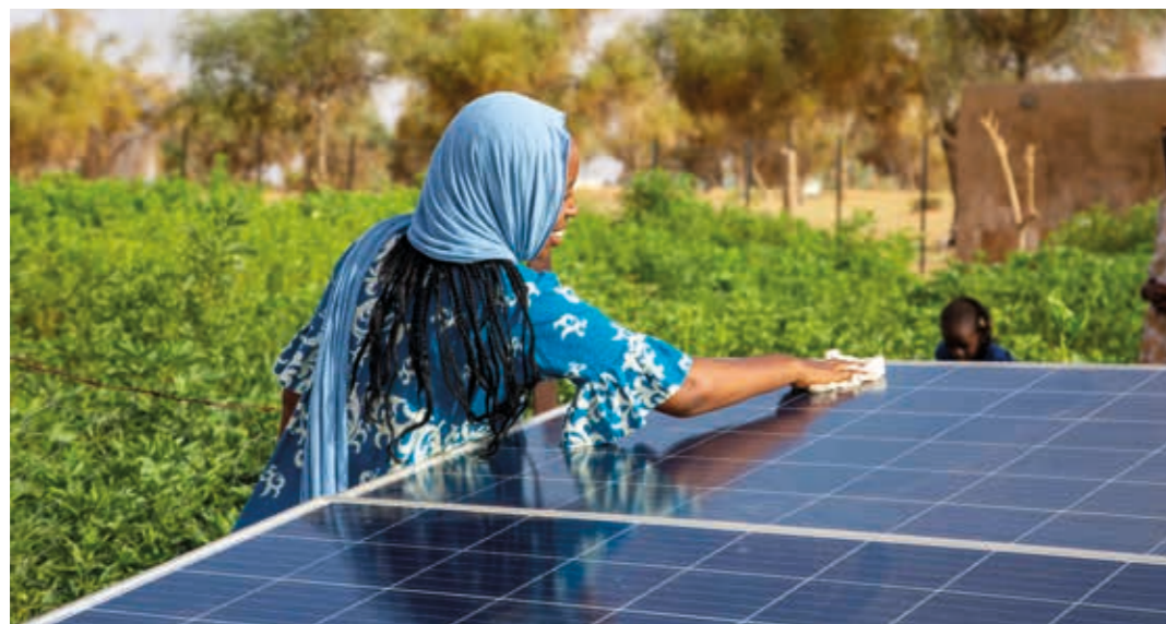
Woman maintaining solar panels of a solar powered water system in Mauritania
