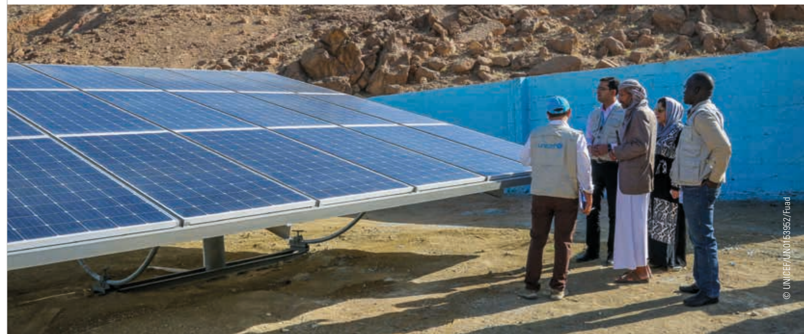
UNICEF staff inspect a newly installed solar system in Sa'ada, Yemen
