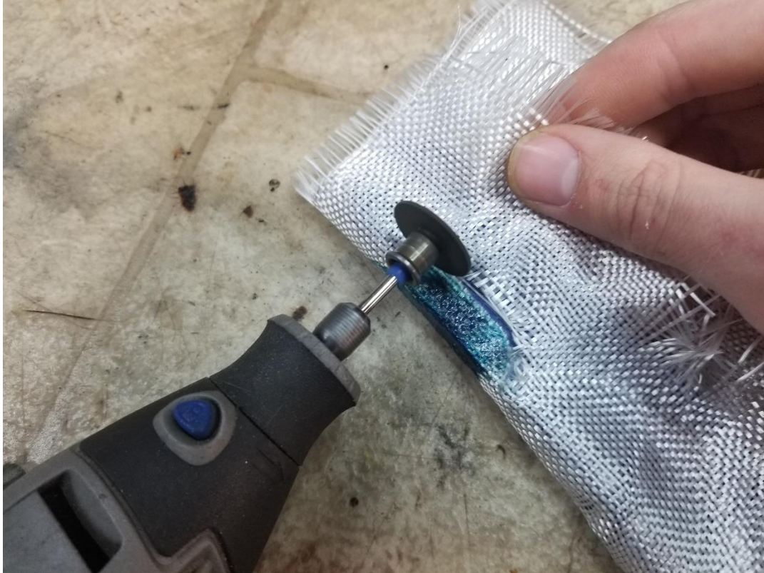
Figure 13: Trim the fiberglass away using a rotary tool. Be careful to not tangle loose strands on the tool!
