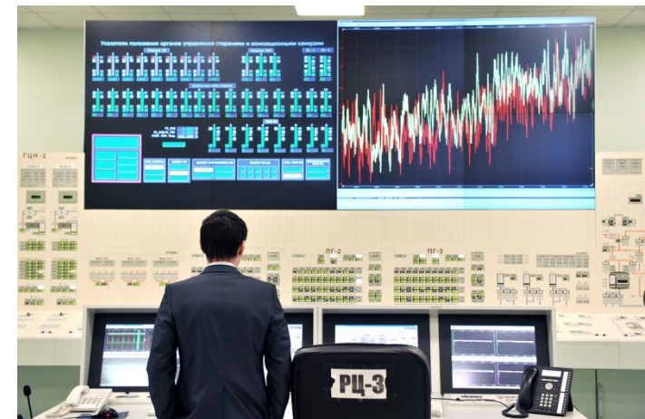
Main control room. Achievement of minimum controllable power.
