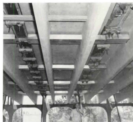
Note ductwork passing through web of tees. This method used to conserve overhead space.
