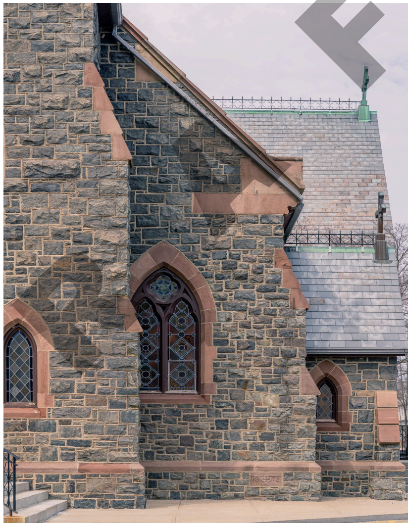
10. Facade detail, showing setbacks and kneelers in gable wall, camera facing north. (See also Graphic 1.)
