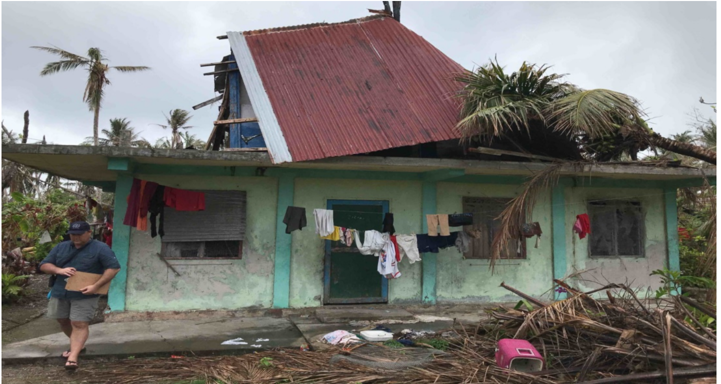
IOM staff Nathan Glancy inspects a damaged house in Chuuk during the JDA. Credit: USAID, 2019
