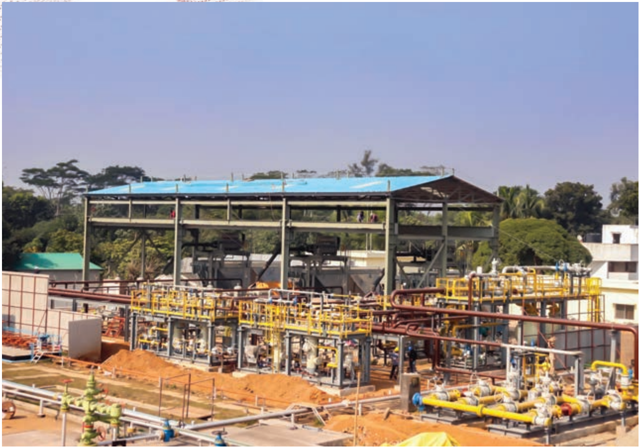
Wellhead compressor of Narshingdi Field of BGFCL
