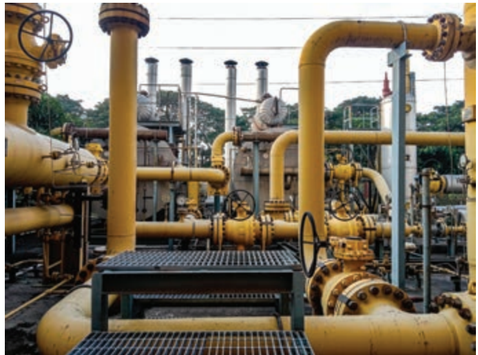
200 MW RMS at Ashuganj of BGDCL
