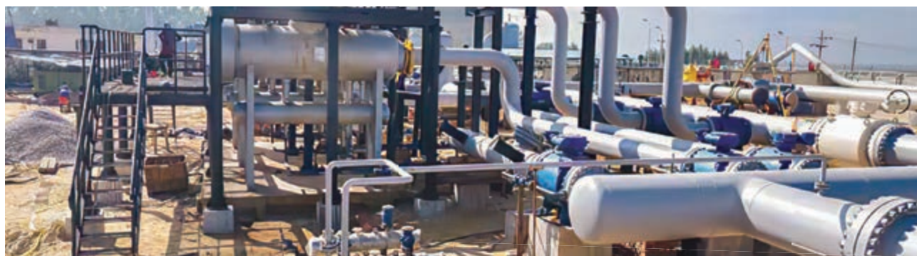
Under construction 1500 million cubic feet capacity metering station at Moheshkhali Zero Point of GTCL
