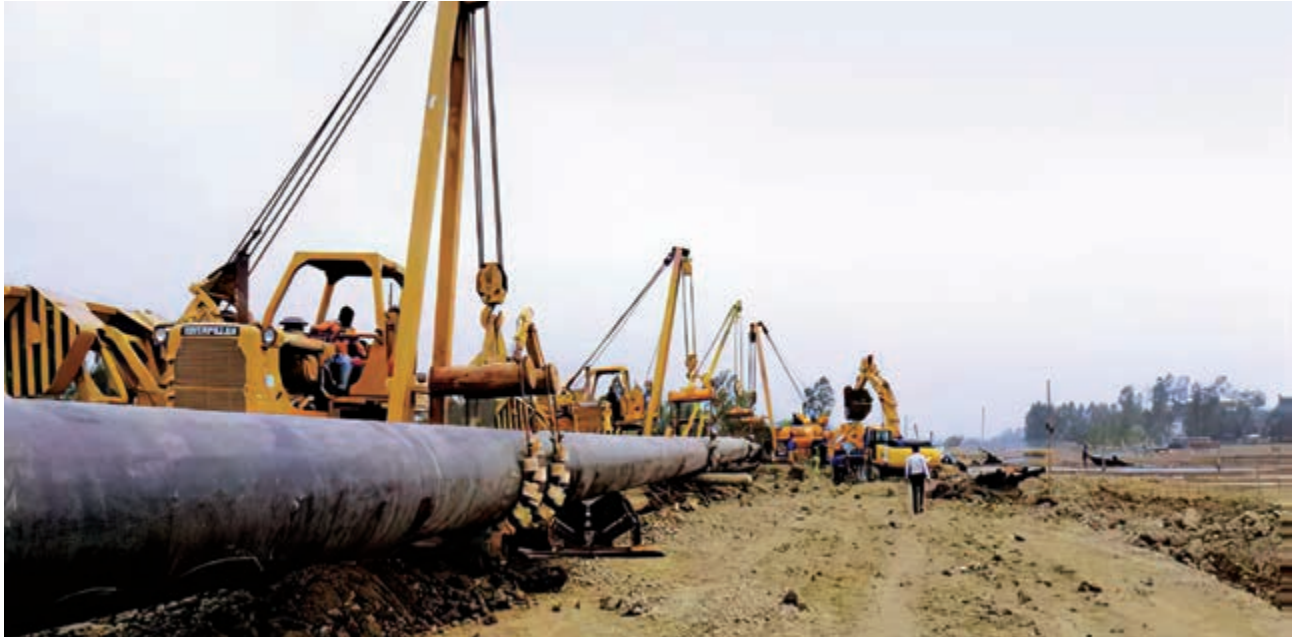
River crossing activities by HDD method under Moheshkhali-Anowara parallel project of GTCL
