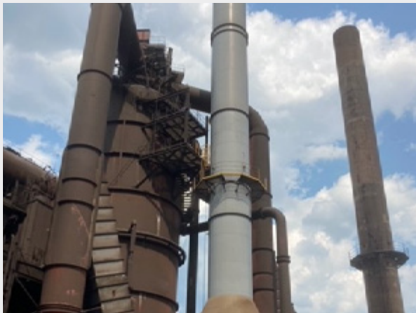
Figure 21. BOP scrubber gas cleaning system.
