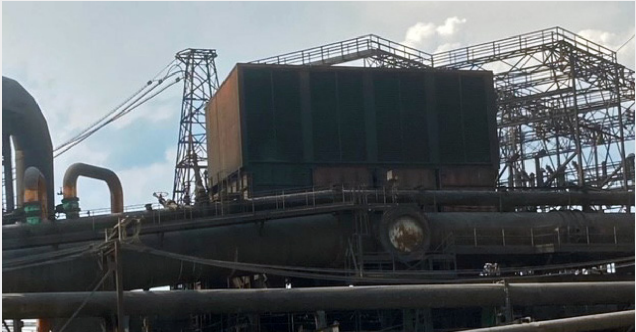
Figure 17. Blast furnace casthouse controls.
