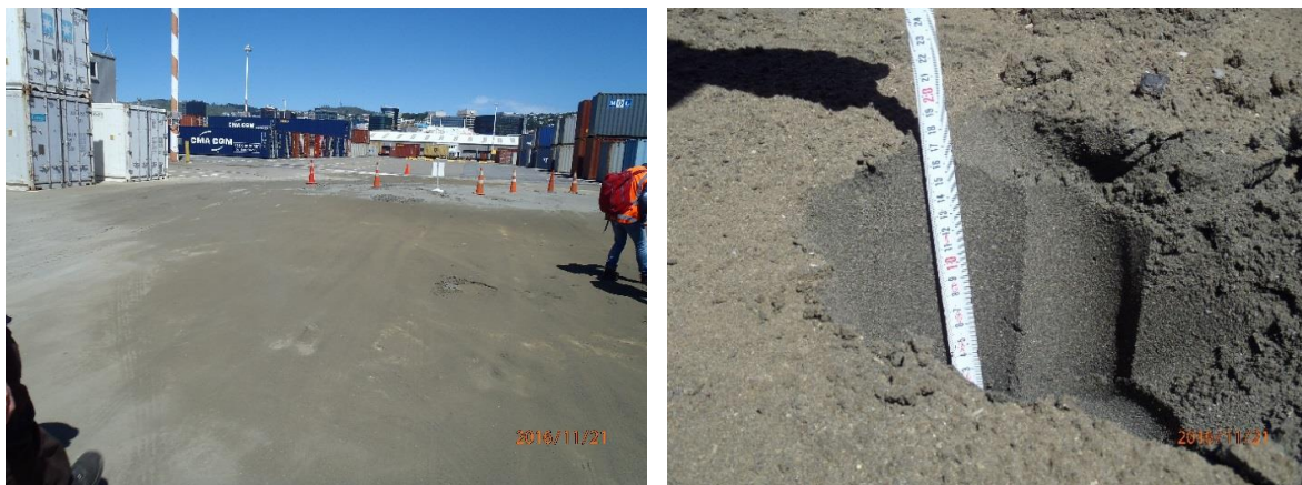
Figure 10: Sandy liquefaction ejecta with trace gravel among area of 1970's end-dumped quarry rock reclamation (i.e., Thorndon Reclamation) at STA 145 and approximately 60 m west of the bulkhead. The ejecta deposit was approximately 170 mm thick at this location. Samples S11 and S12 were collected here (S41.279067° E174.788792°, taken on 21NOV2016).
