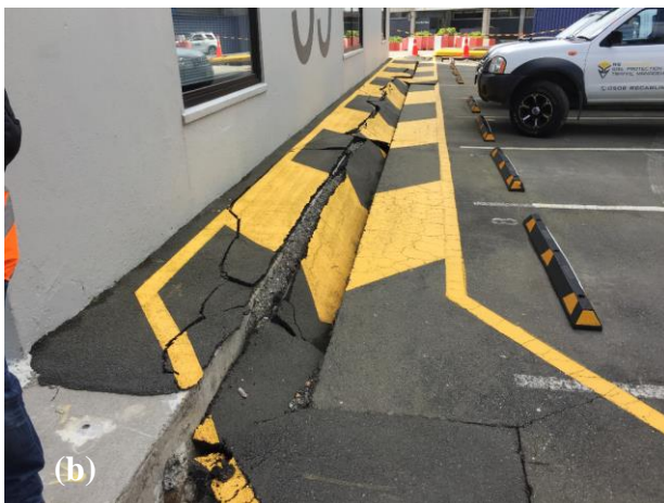
Figure 33: (a) Southeast side of Building S39 and a buried segment of the Fryatt Quay Wharf deck parallel to the building. Fill to the south of the buried mass concrete seawall/wharf settled 220 mm relative to the pile-supported building and wharf deck. ( S41.277984^{\circ} E174.785776^{\circ} , 22NOV16), and (b) looking southeast along southwest wall of Building S39. Fill settled approximately 190 mm relative to pile-supported building at the northwest corner of the building (shown on lower left corner of photo), and magnitude of settlement decreased south-eastward along this wall. ( S41.277994^{\circ} E174.785467^{\circ} , 17NOV16).
