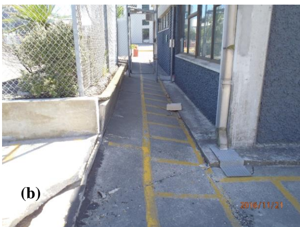
Figure 25: (a) Uniform settlement of CPH building which is founded on shallow foundations that apparently displaced downward the same amount as the surrounding fill. This photo is looking northeast at the southwest corner of the building. (S41.278395° E174.785639°, taken on 21NOV16). (b) Uniform settlement (230–260 mm) of the building relative to ground supported on the buried precast seawall that ran parallel to the bulkhead of partially demolished Pipitea Wharf. Looking north along western wall of CPH building. The perimeter walkway slopes down towards the building at 11 degrees over 1.35 meters. (S41.278395° E174.785639°, taken on 22NOV16).
