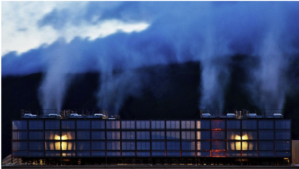
Figure 6.29 Steam rising from the cooling towers that transfer heat to the air from the water used to cool equipment.
