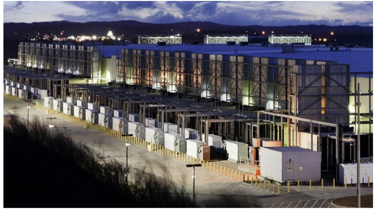
Figure 6.25 This image shows transformers, switch gear, and generators in close proximity to a WSC.
