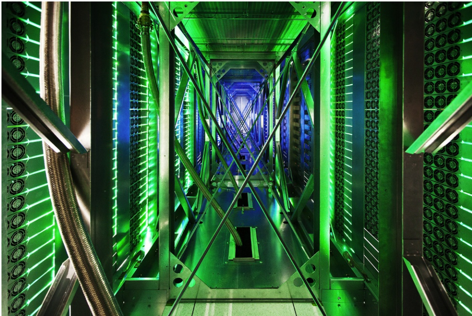
Figure 6.27 Hot aisle in a Google data center, which is clearly not designed to accommodate people.
