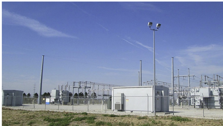
Figure 6.24 An on-site substation.
