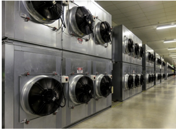
Figure 6.28 The cool air blows into the room containing the aisles of servers. The hot air goes through large vents into the ceilings where it is cooled before returning to these fans.
