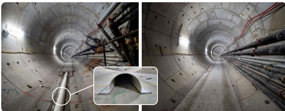
A PVC half-pipe supports drainage within the tunnels (pictured left). The invert slab creates the base for the rail and sleepers (pictured right)
