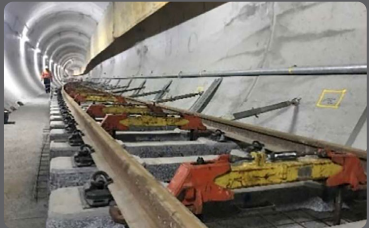
Track adjustment system used to set rail to design line and level
