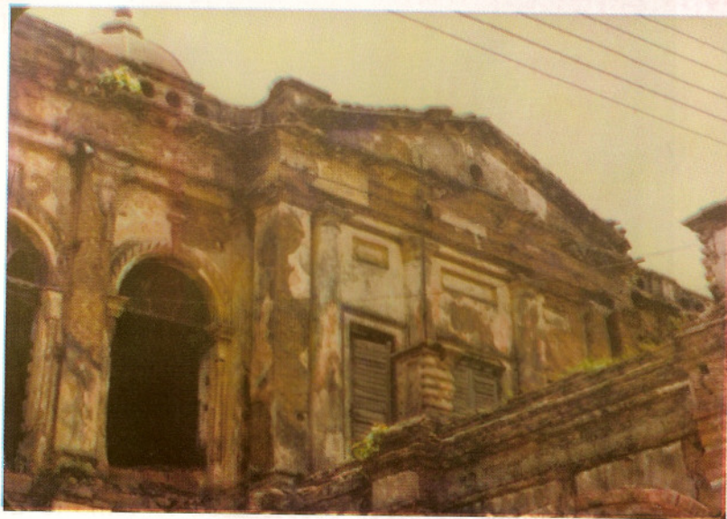
No.10, Dilapidated condition of Ahsan Manzil, 1986, Pediment on north porch
