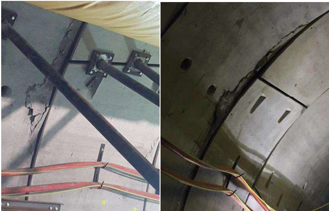
Figure 2 - View of Ring 117 (left) and Ring 120 (right) both with tension cracks and lips
