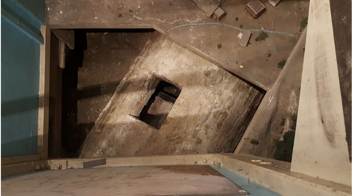
Figure 2. Exposed Zanja Madre conduit in the Avila Adobe Interpretive Center, El Pueblo de Los Angeles Historical Monument. Image courtesy of the Los Angeles Department of Water and Power.
