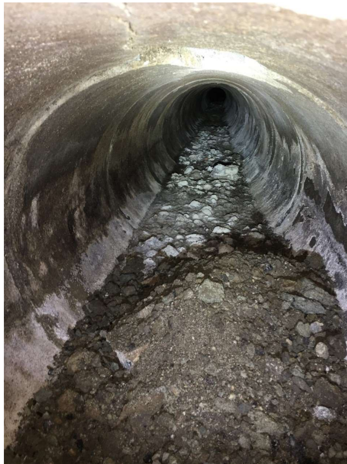
Figure 7. Zanja No. 8-R beneath Flower Street, view southwest. Image courtesy of AECOM.
