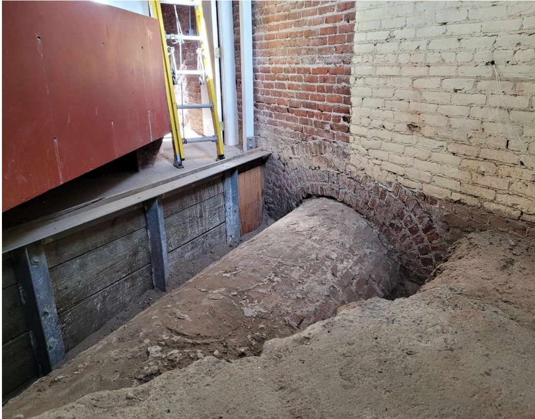
Figure 5. Zanja Madre Segment Beneath the 1909 Hammel Building. Image courtesy of the Los Angeles Department of Water and Power.
