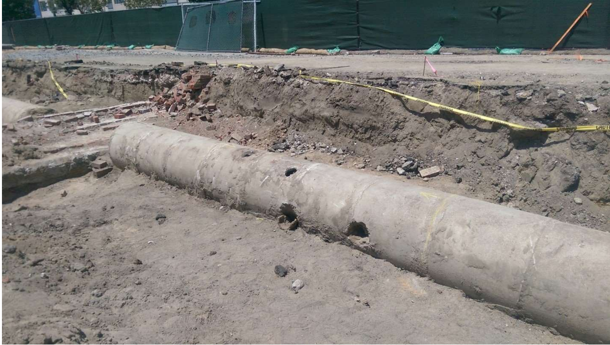
Figure 6. Zanja No. 3 Concrete Pipe broken by 1897 commercial building foundation, view southwest. Image courtesy of AECOM.
