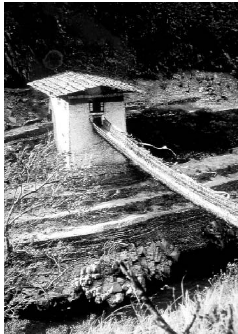
Fig. 36: The former Tashigang Chakzam across the Drangme Chhu. Photo: Fritz von Schulthess.
