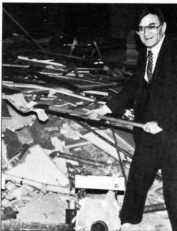
ABC Radio programming vice president Rick Sklar breaks ground for new studios intended to house Superadio, a satellite-delivered format. But the poor economic climate forced Superadio down the drain two weeks prior to its July 1 debut. Also indefinitely delayed was the United Stations' country satellite network.
