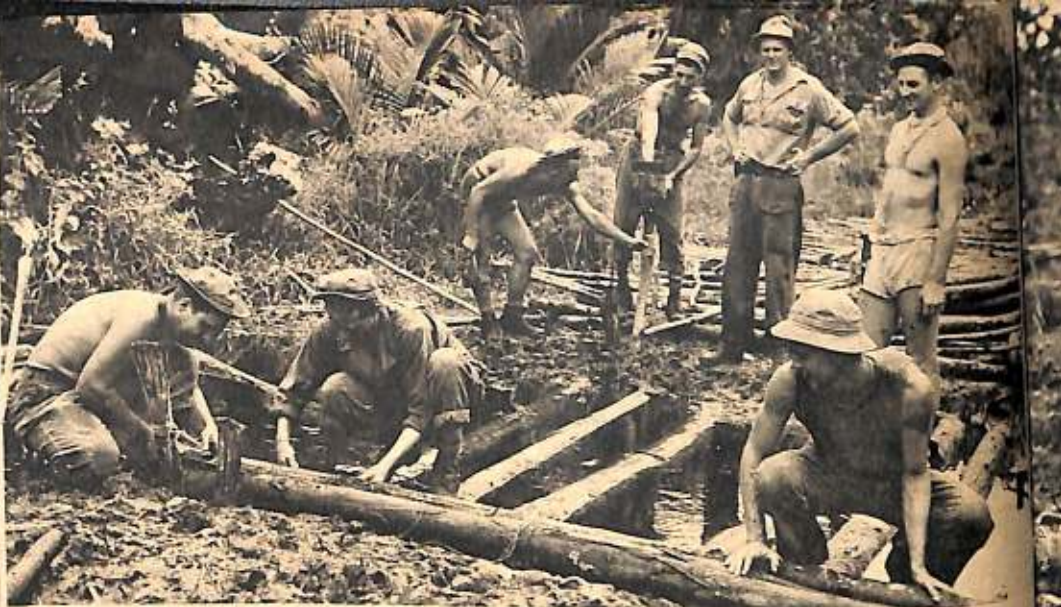
THE ENGINEERS. These GIs are building a corduroy road of coconut-palm logs, so that Army supply transport won't bog down in the tropical mud.
