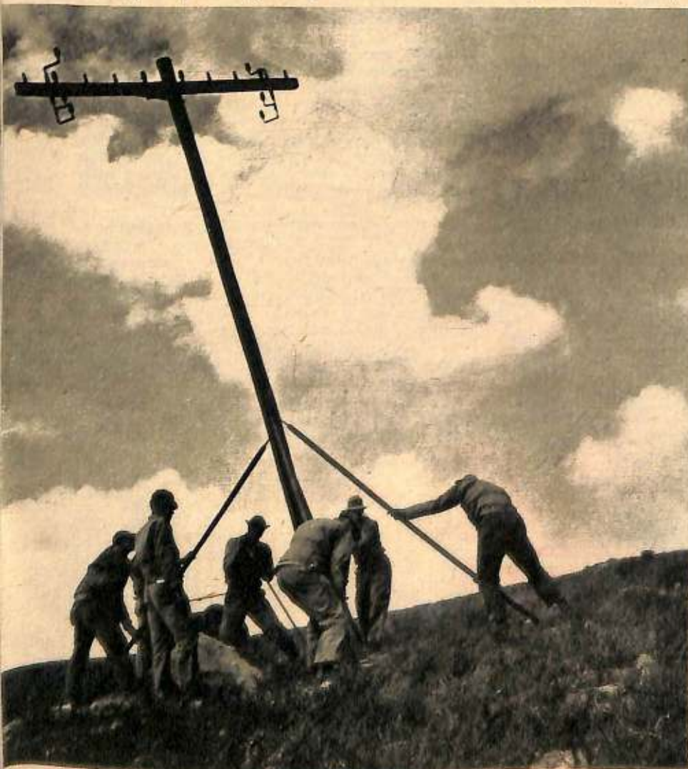
ON LAND a crew of pole setters raise one in place near a base HQ. A wire crew follows. Such outfits have set new records for speed.
