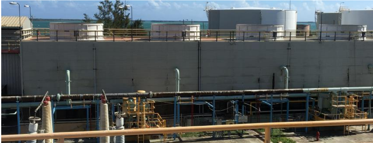
Figure 2-7 — Closed Cooling Tower for Thermal Units 1 and 2
