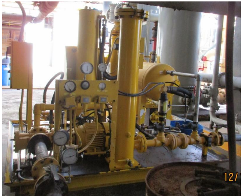
Unit 2 STG lube oil filtering skid.
