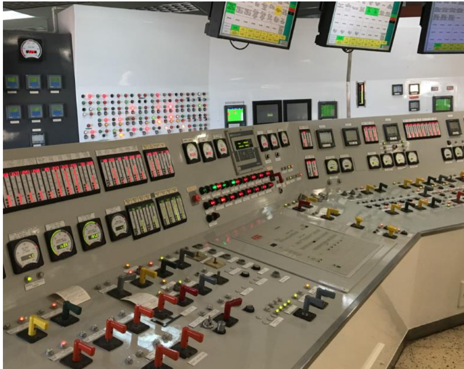
Figure 3-33 — Control Room Units 1-2
