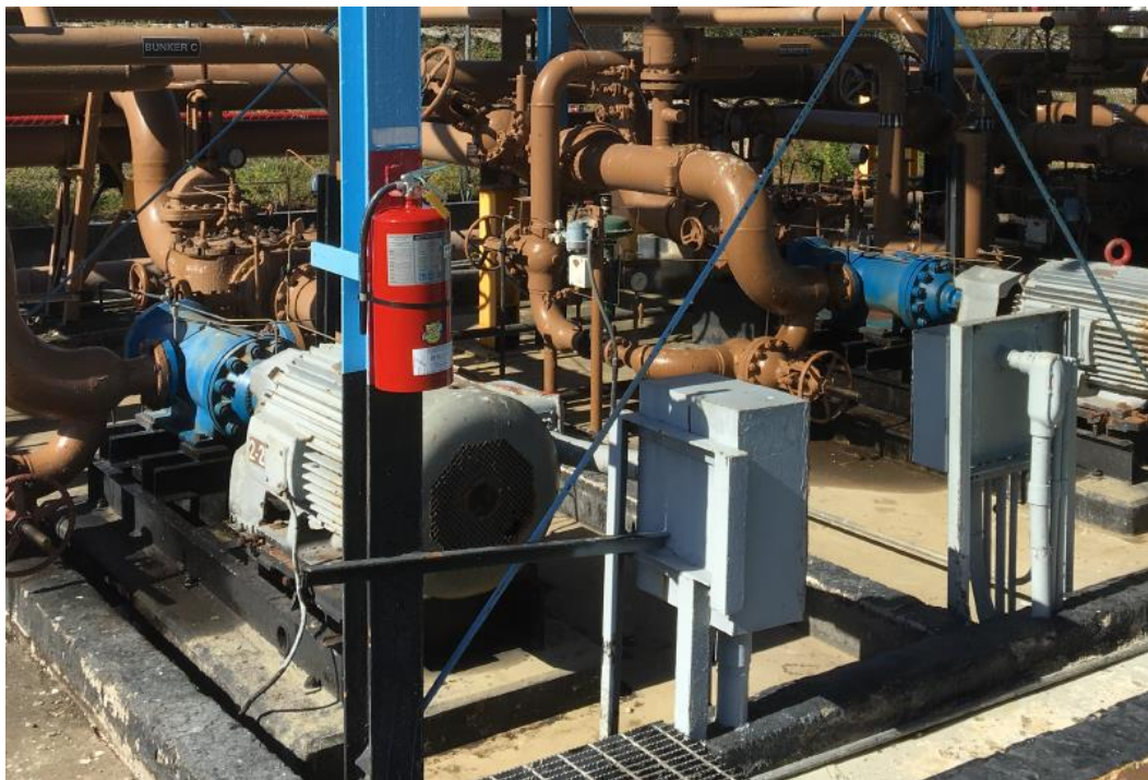
Figure 3-16 — HFO Forwarding Pump
