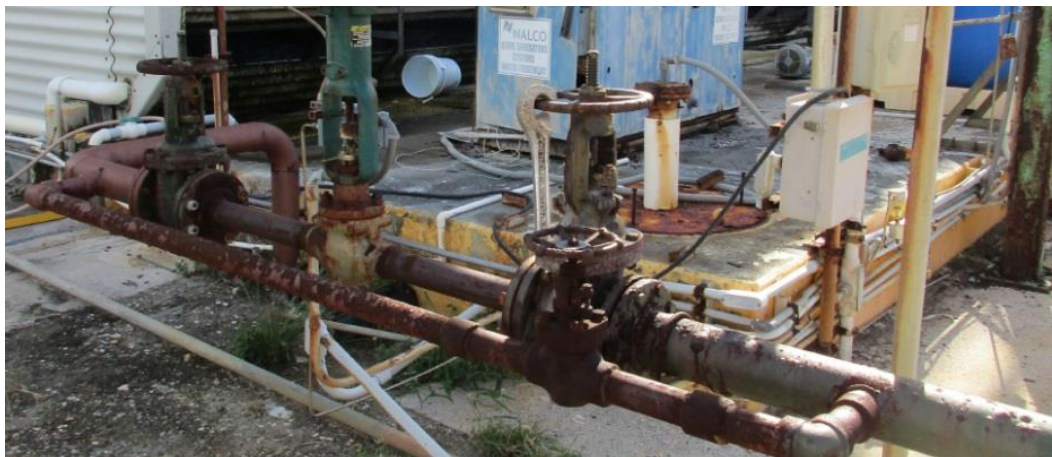
Figure 3-24 — Combined-Cycle Closed Cooling Water Tower
