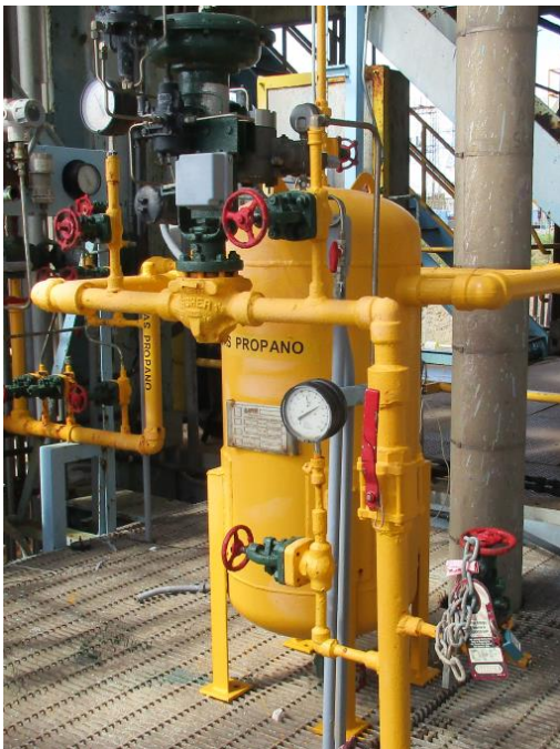
Unit 1 Propane tank, piping, and valves.
