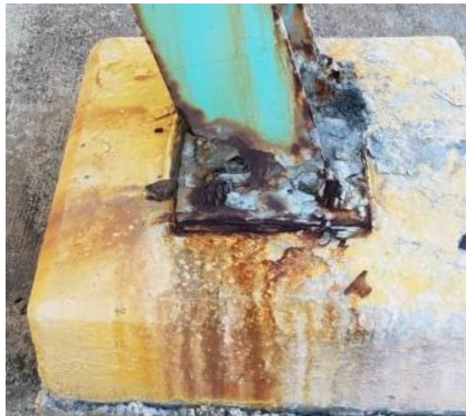
Figure 3-40 — Corrosion of Gantry Crane Structural Steel at Combined-Cycle Plant
