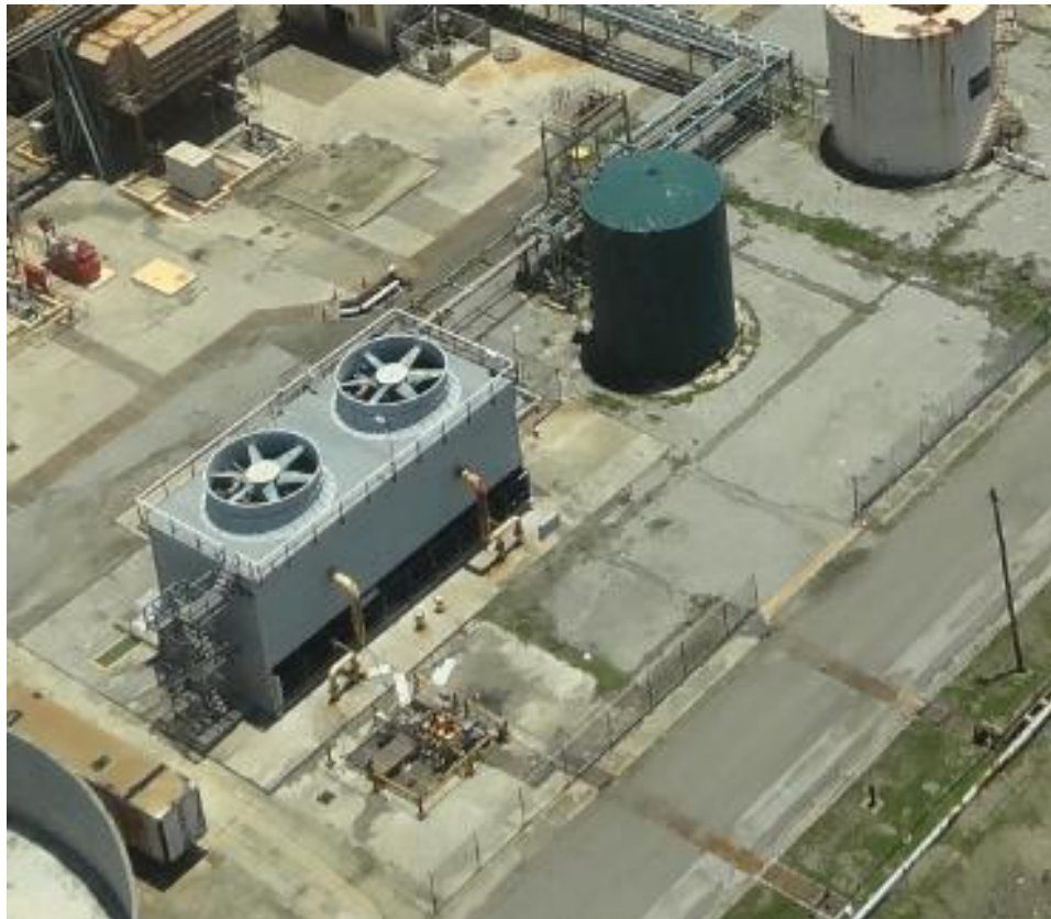
Figure 2-8 — Closed Cooling Tower for Combined Cycle Unit
