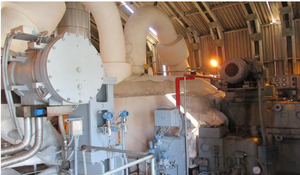
Figure 3-1 — Unit 1 STG HP Section with Turning Gear
