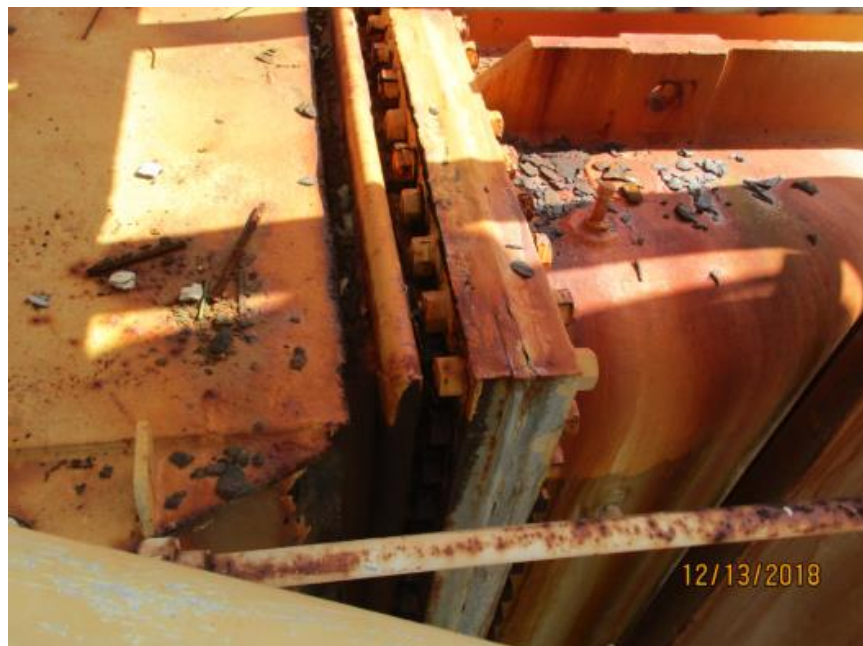
One of the STAG 1 condensers with waterboxes coated on the inside in 2017.
