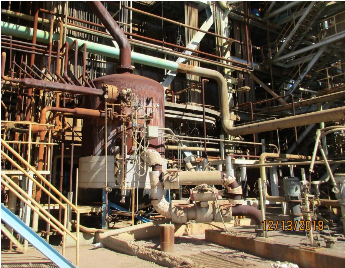
Figure 3-5 — Unit 2 Boiler Blowdown Tank
