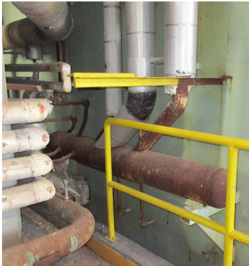
Figure 3-30 — Corroded Drain Lines into Unit 2 Condenser
