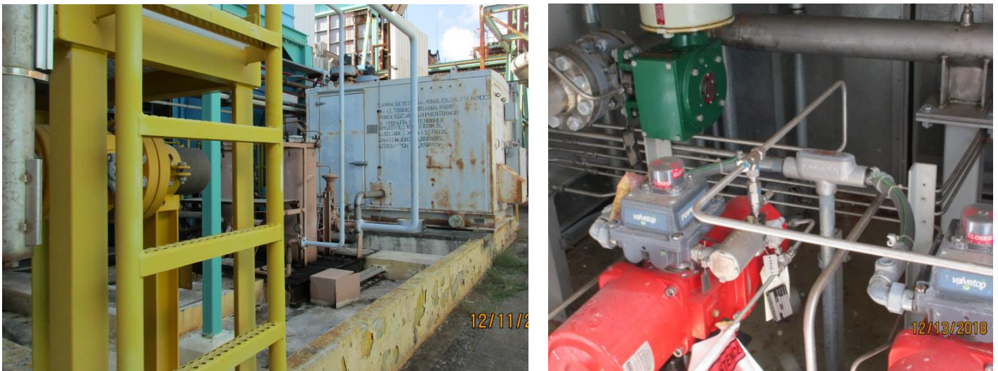
Figure 3-42 — Natural Gas Delivery Components Installed at CC Units
