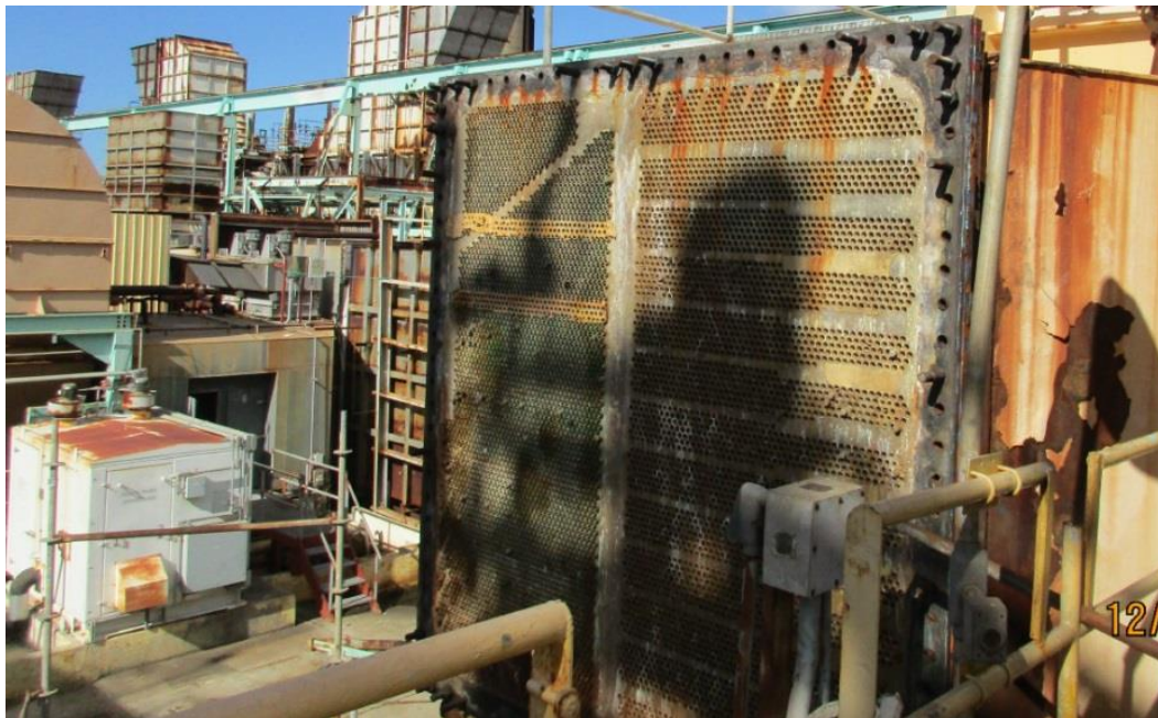
Figure 3-32 — Combined-Cycle STAG 2 Condenser
