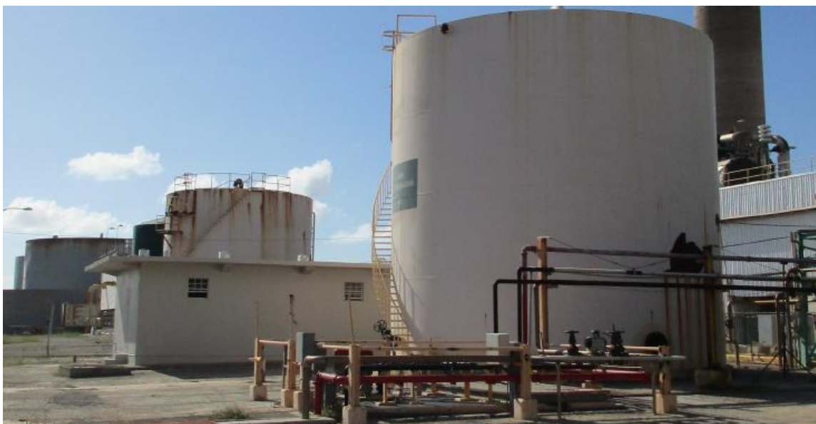
Figure 3-22 — Demineralized Water and Condensate Tanks at CC Unit
