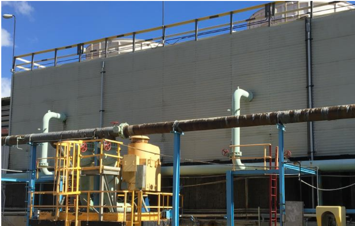
Figure 3-23 — Closed Cooling Tower, Units 1 and 2
