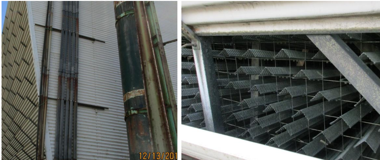
Figure 3-28 — Seawater Cooling Tower – STAG 1
