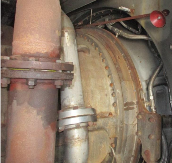
GT1-4 compressor casing
