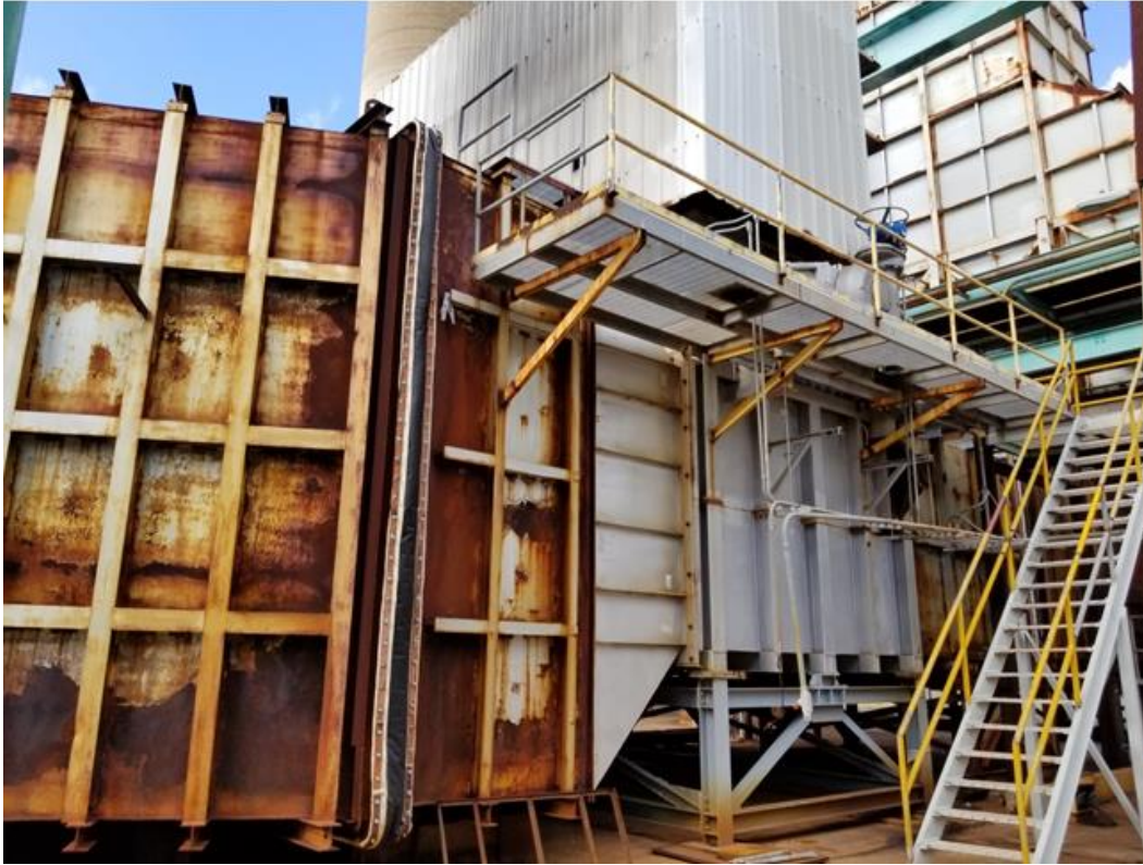
Figure 3-11 — GT Discharge Duct Diverter Damper and Stack
