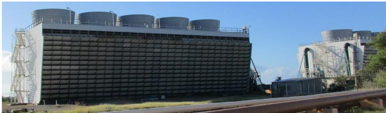
Figure 2-6 — Combined-Cycle Seawater Cooling Towers
