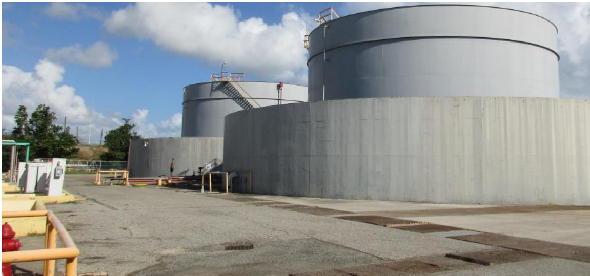
Figure 2-10 — No. 2 Fuel Oil Tanks at Combined Cycle Unit
