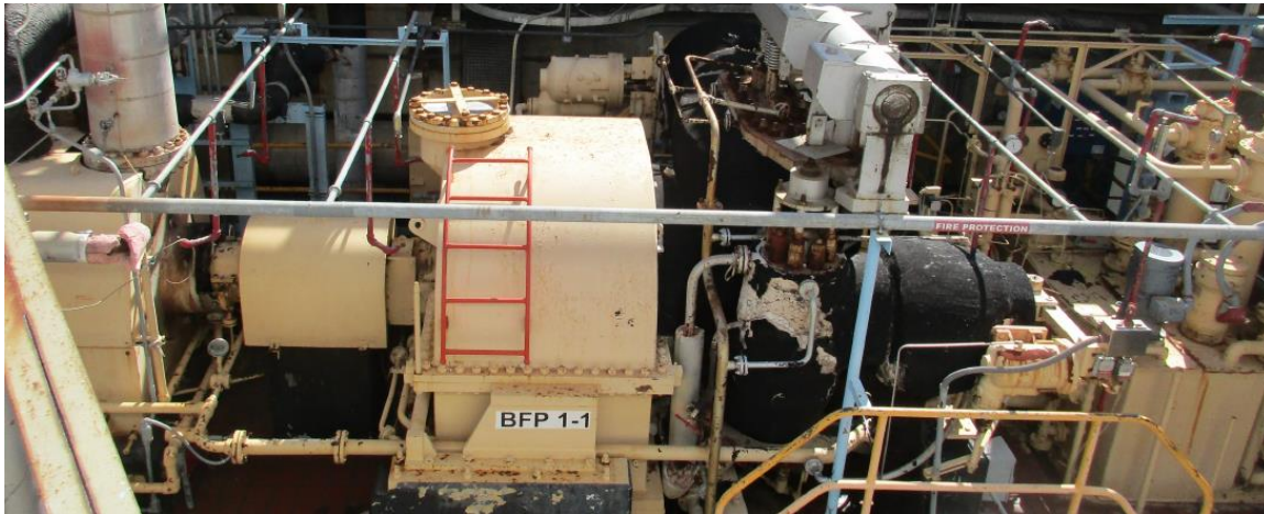
Figure 3-2 — Steam-Driven BFP, Unit 1
