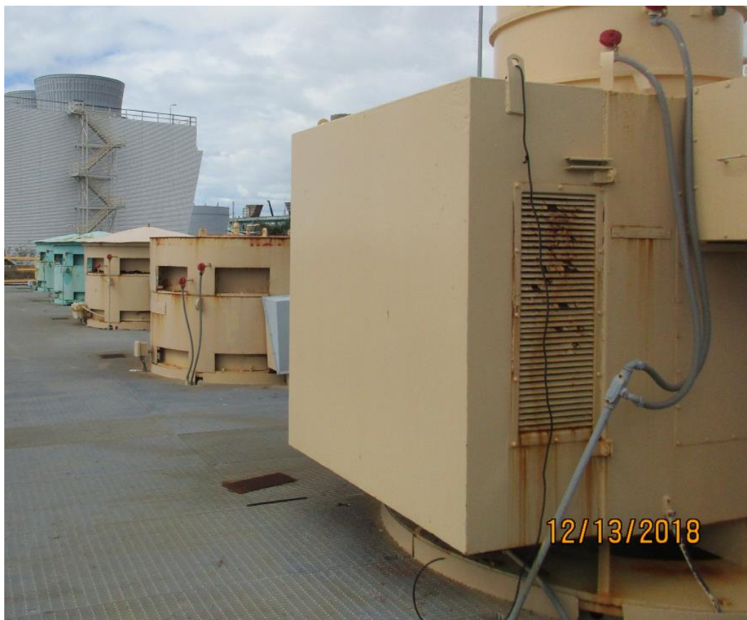
Figure 3-27 — Circulating Water Pumps
