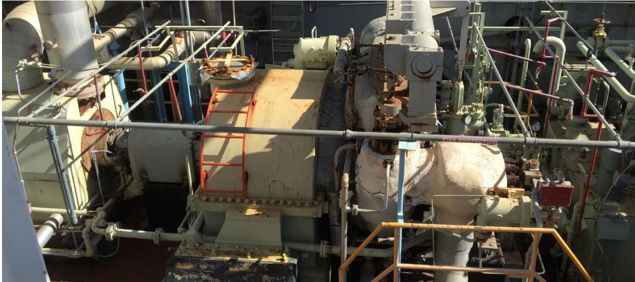
Figure 3-4 — Steam-Driven BFP Unit 2
