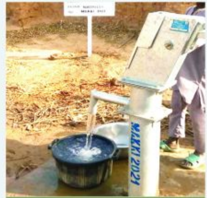
One of the Hand pumps constructed under the CSR project
