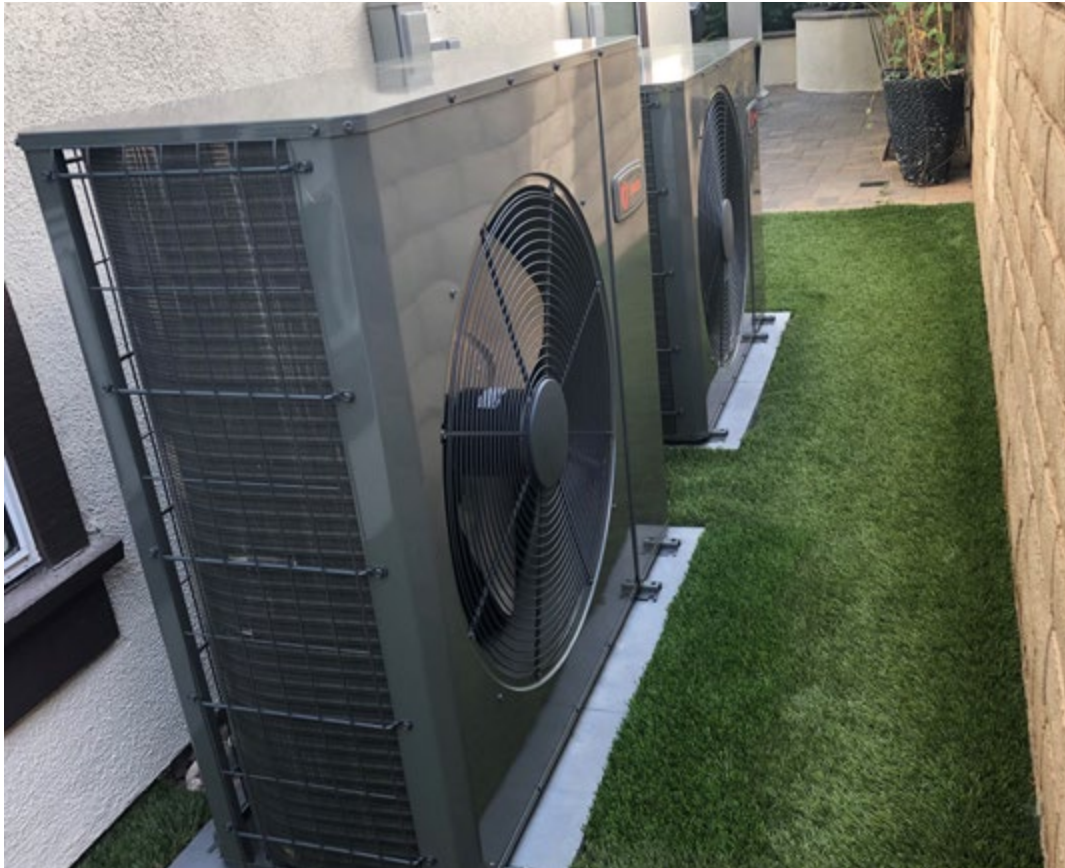
New condensing units for a dual heat pump HVAC system that both heats and cools using electricity. These types of systems can be three to four times more efficient than a gas furnace and a traditional stand-alone air conditioning system.
