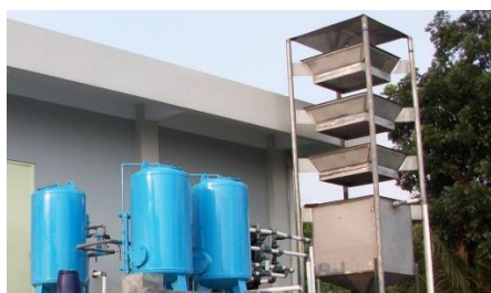
Gambar 8. Water treatment plan Sumber: Hasil survei, 2016
