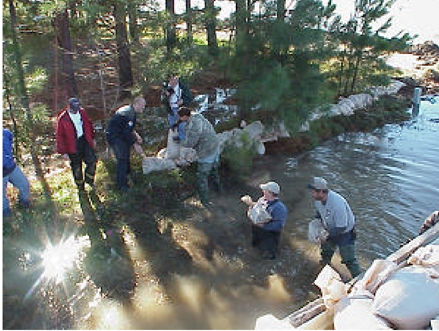
Sandbagging was necessary to hold back flood waters on Jackson County Road 82 (north of Grubbs) on 12/18/2001.
