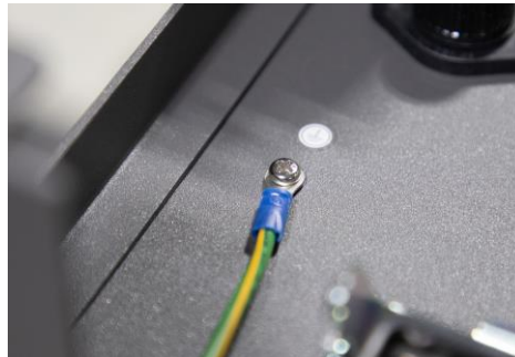
Figure 22: Grounding position for the control box
