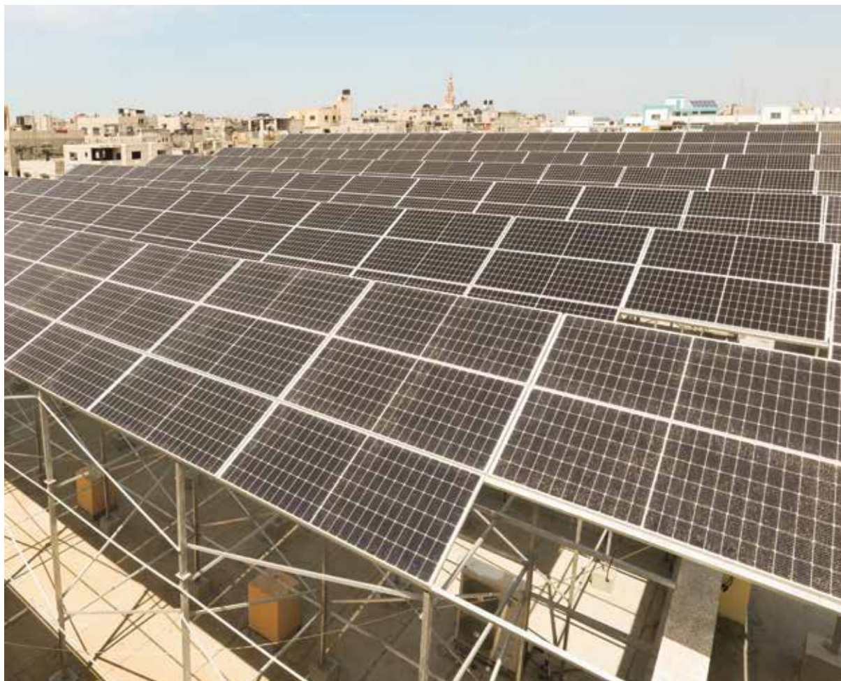
Figure 1: Example of Existing Installation at Nasser Hospital
