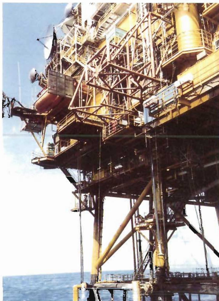
Plate 10(b) The north-west corner of the platform, showing the Chanter riser gantry. The gantry is the two structures, one ending in a triangular shape and the other in a rectangular one, projecting from the 68ft level. Also shown is the 20ft level and the navigation aid platform at the north-west corner of the 68ft level.
