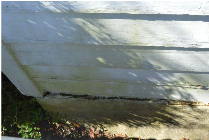
Figure 115. (Photo 98) Microclimate behind accessibility ramp and bush on southeast corner of structure; foundation extends past siding, creating an opportunity for water to enter the building
