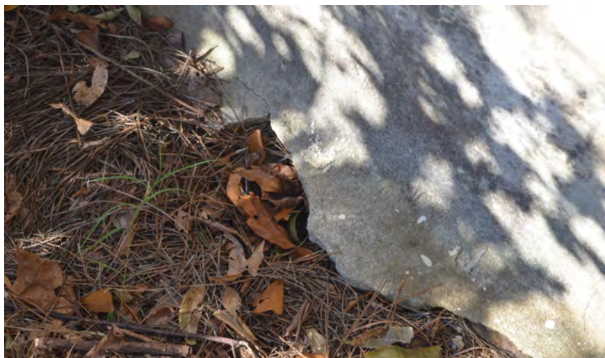
Figure 117. (Photo 100) Hole on northeast corner of east facade that opens to the basement
