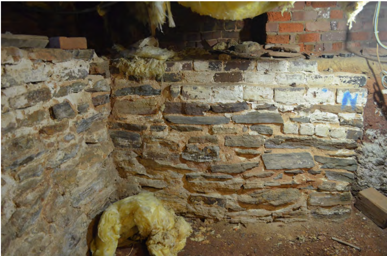
Figure 31. (Photo 21) North and west walls of dugout basement, constructed with field stone and historic brick and previously whitewashed
