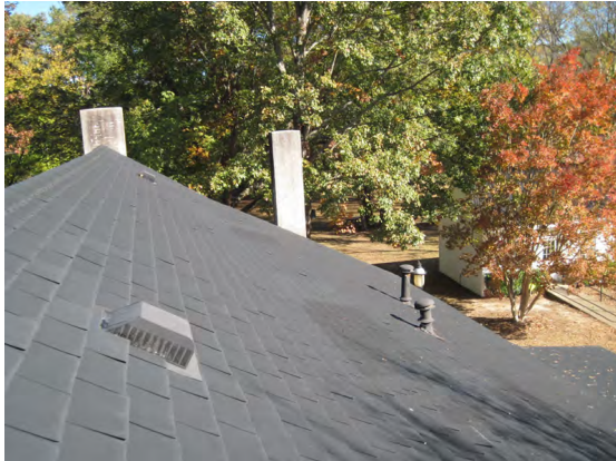
Figure 28. (Photo 18) View of architectural shingle on ridgeline and east slope of roof
