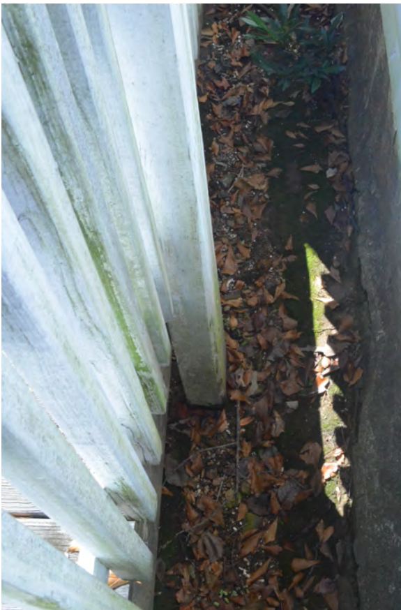
Figure 114. (Photo 97) Large microclimate of microbial growth and damp ground behind accessibility ramp
