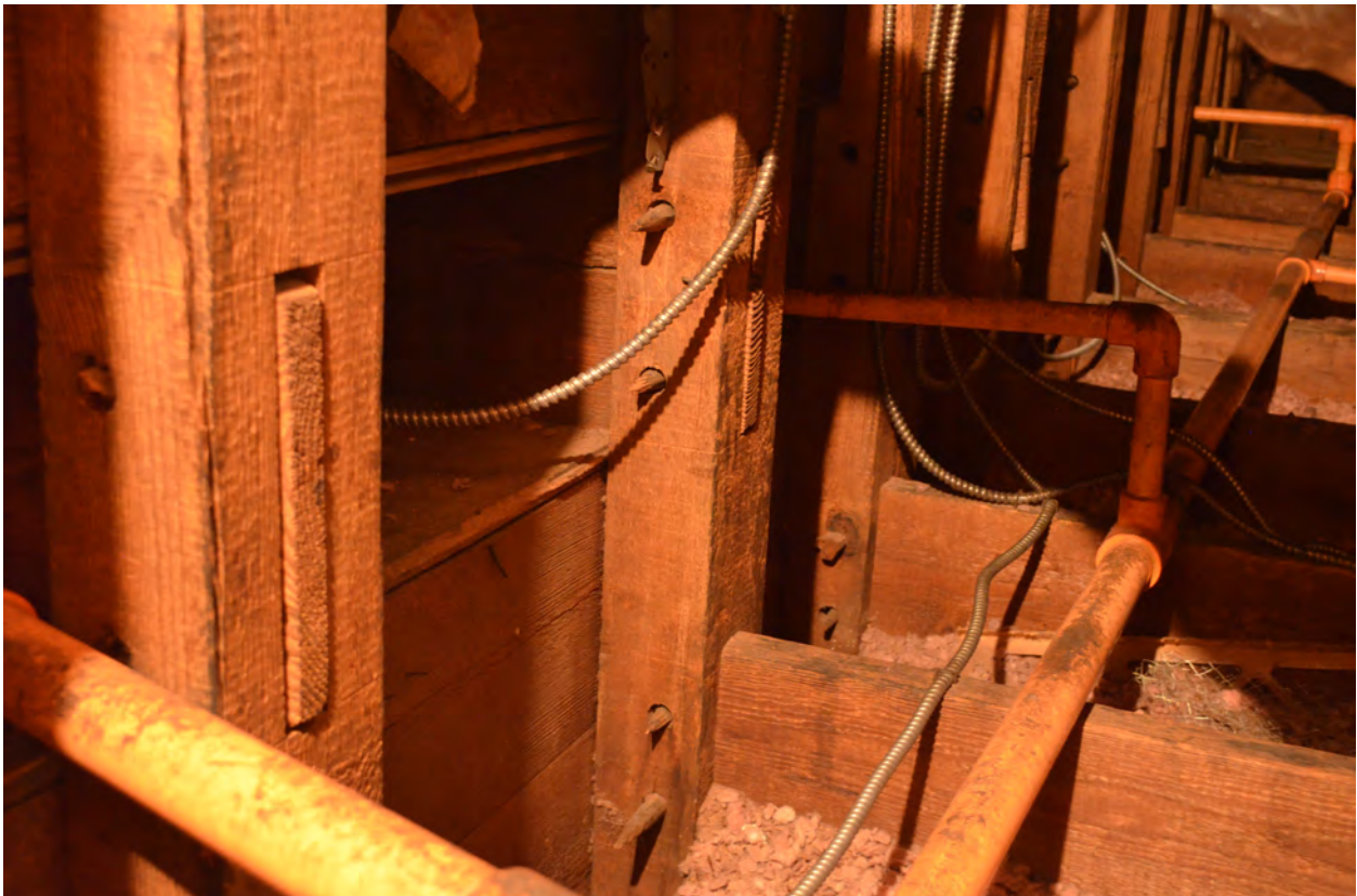
Figure 84. (Photo 71) First floor ceiling joists visible from room 204, Large studs support the floor and ceiling joists, which are joined with pegged mortise and tenon
