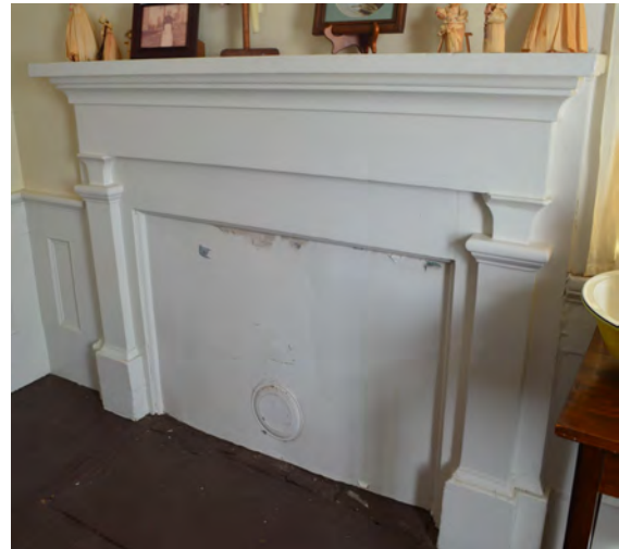
Figure 45. (Photo 33) Sealed firebox in Room 105
