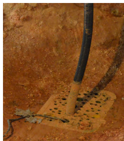
Figure 34. (Photo 34) Sump pump in earth floor of dug out area
