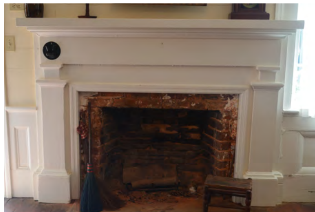
Figure 46. (Photo 34) Added white trim to the front façade of the firebox in Room 102
