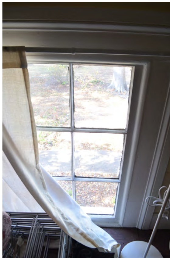
Figure 79. (Photo 66) W20 and W21 on east wall are set directly in contact with the floor
