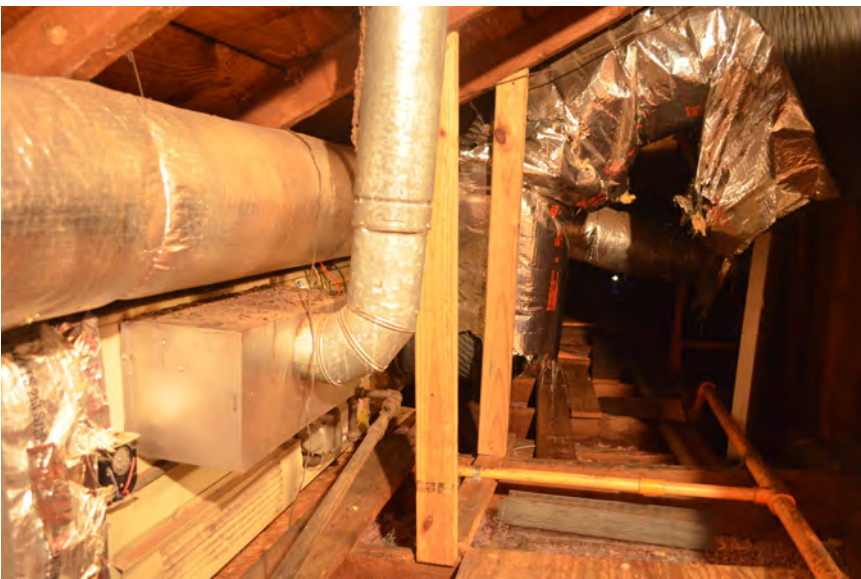
Figure 91. (Photo 76) Old furnace in room 204, servicing the second floor.
