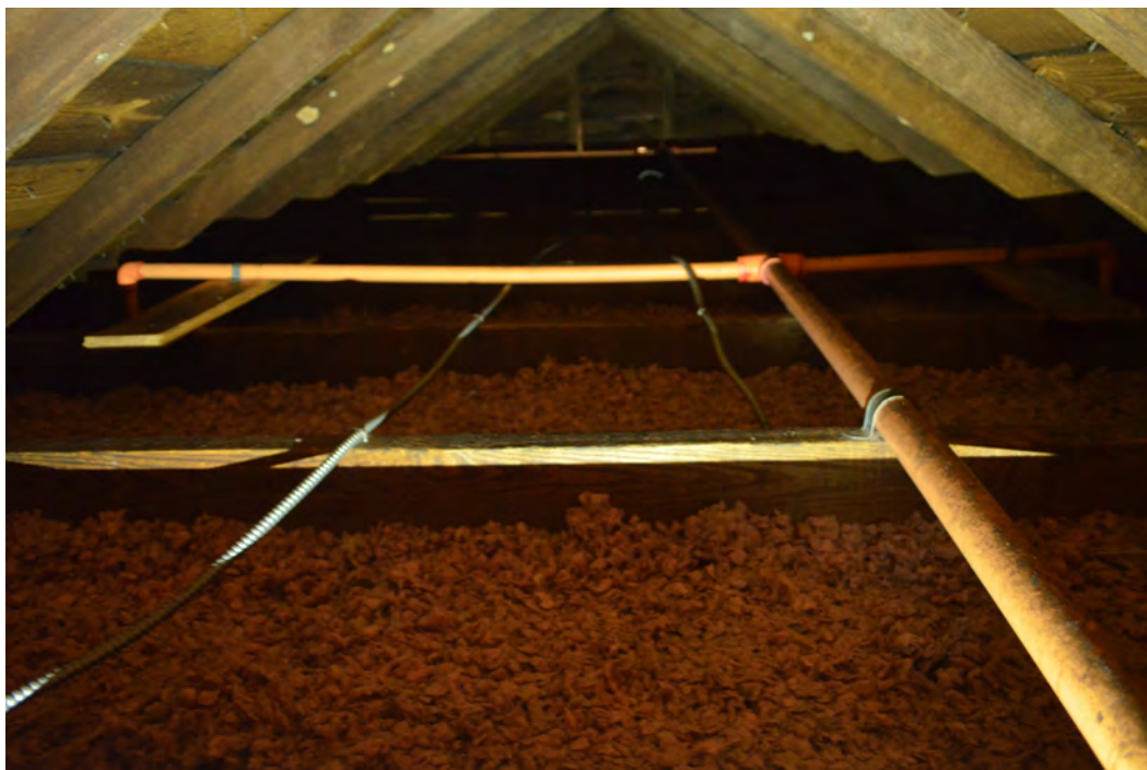
Figure 90. (Photo 75) Sprinkler system, modern electrical conduit, and fiberglass insulation visible in room 301.
