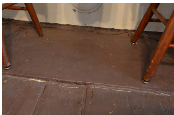
Figure 51. (photo 39) Painted dark brown floor near the fireplace on the north wall in Room 105
