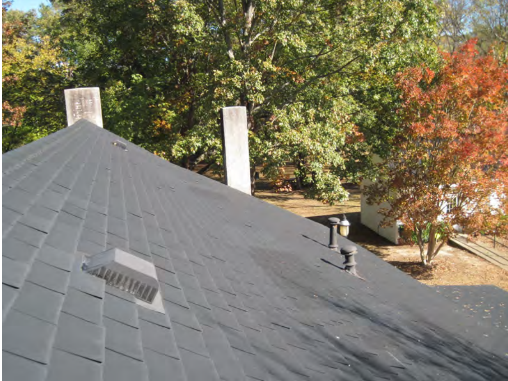
Figure 17. (Photo 11) View of architectural shingle on ridgeline and east slope of roof
