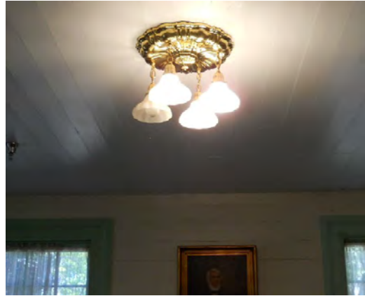
Figure 43. (Photo 31) Light fixtures in room 103
