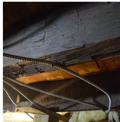
Figure 33. (Photo 23) Framing for first floor and original hand hewn sills visible from basement
