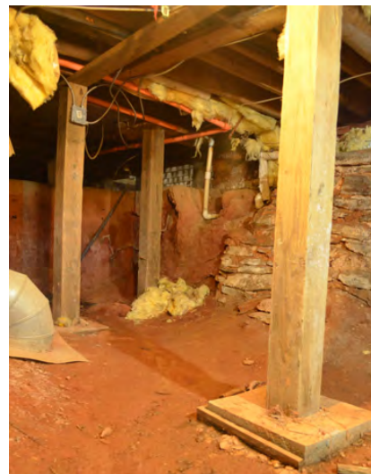
Figure 32. (Photo 22) Modern 6" x 6" wood posts on modern concrete footers support floor joists
