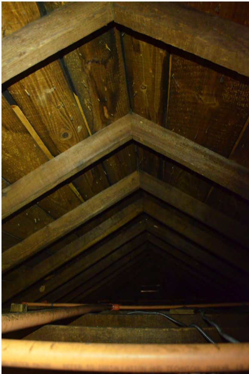
Figure 88. (Photo 74) Looking south, Rafters in room 301; no ridge board or joinery at peak
