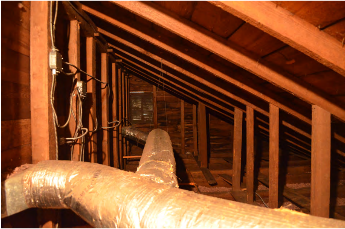
Figure 85. (Photo 72) Lowered vent and exposed weatherboard on the north gabled end house appears to be historic
