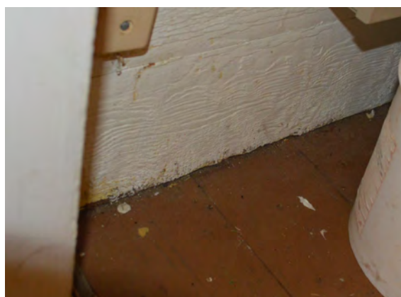
Figure 53 (Photo 41) Room 101, the interior of the staircase closet shows an ochre painted floor.
