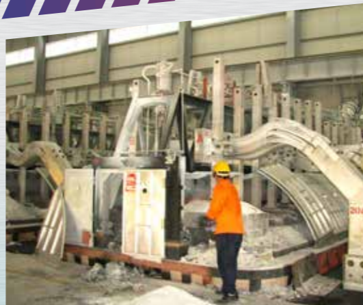
14 November, 2012 The initial commissioning phase of Press Metal Bhd's aluminium smelting plant in Samalaju Industrial Park
