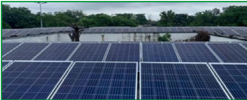
Roof-Top Solar Project of ECL
