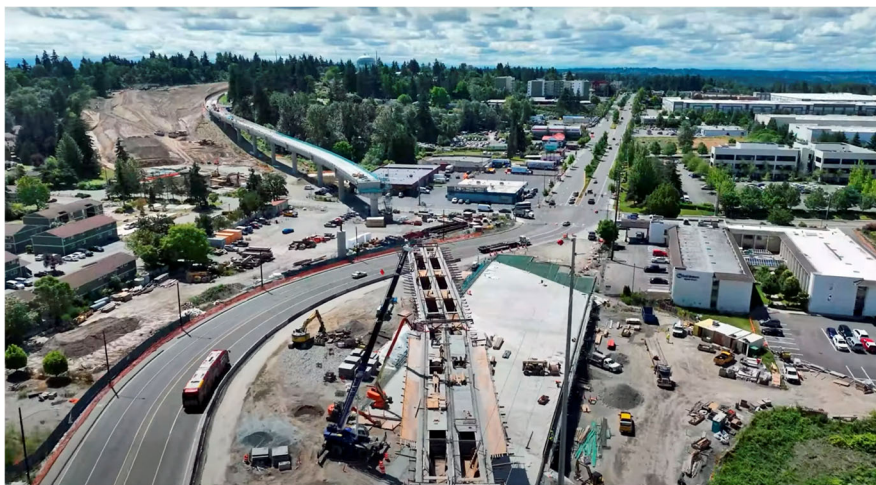
Uploaded quarterly flyover video to YouTube for sharing with AHJs and the public.
