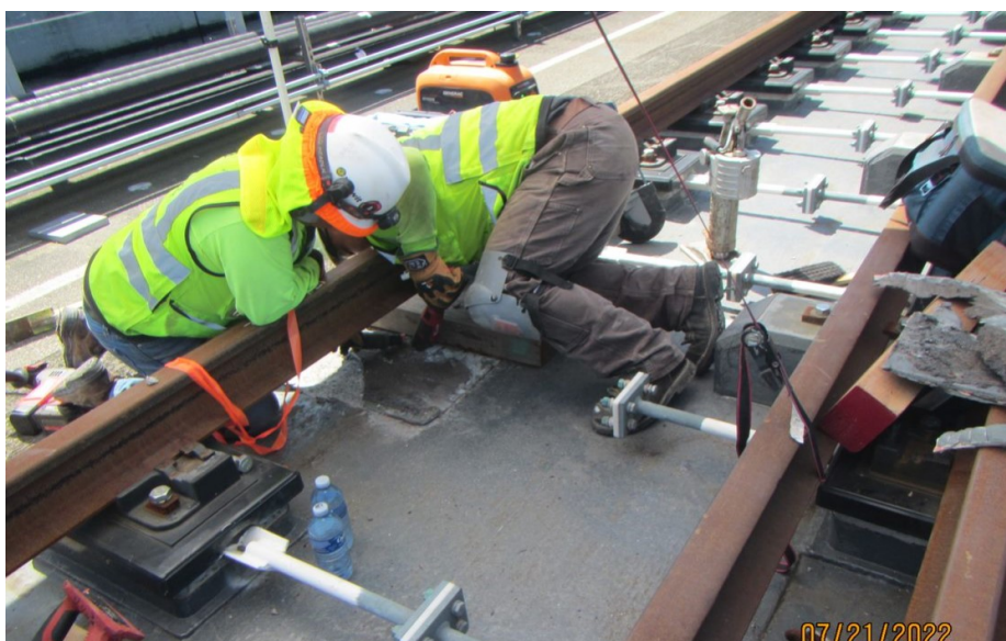
E130 Seattle to South Bellevue: Removal of dual block plinths on I-90 floating bridge segment for testing.
