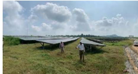
10MW Solar plant at BHPL Region.
