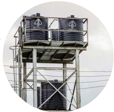
Borehole constructed for 1000 people in Ajoki and Ajamimogha Communities of Edo State
