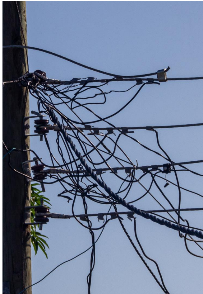
Distribution network installations, Havana
