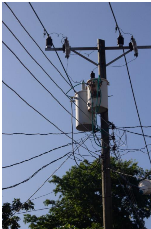
Distribution network transformer
