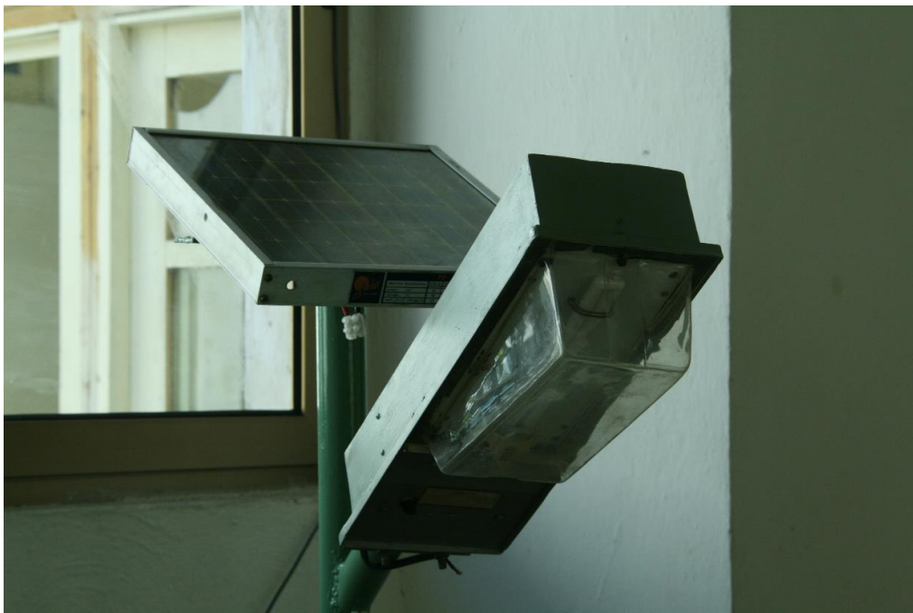
Street lighting with a photovoltaic panel
