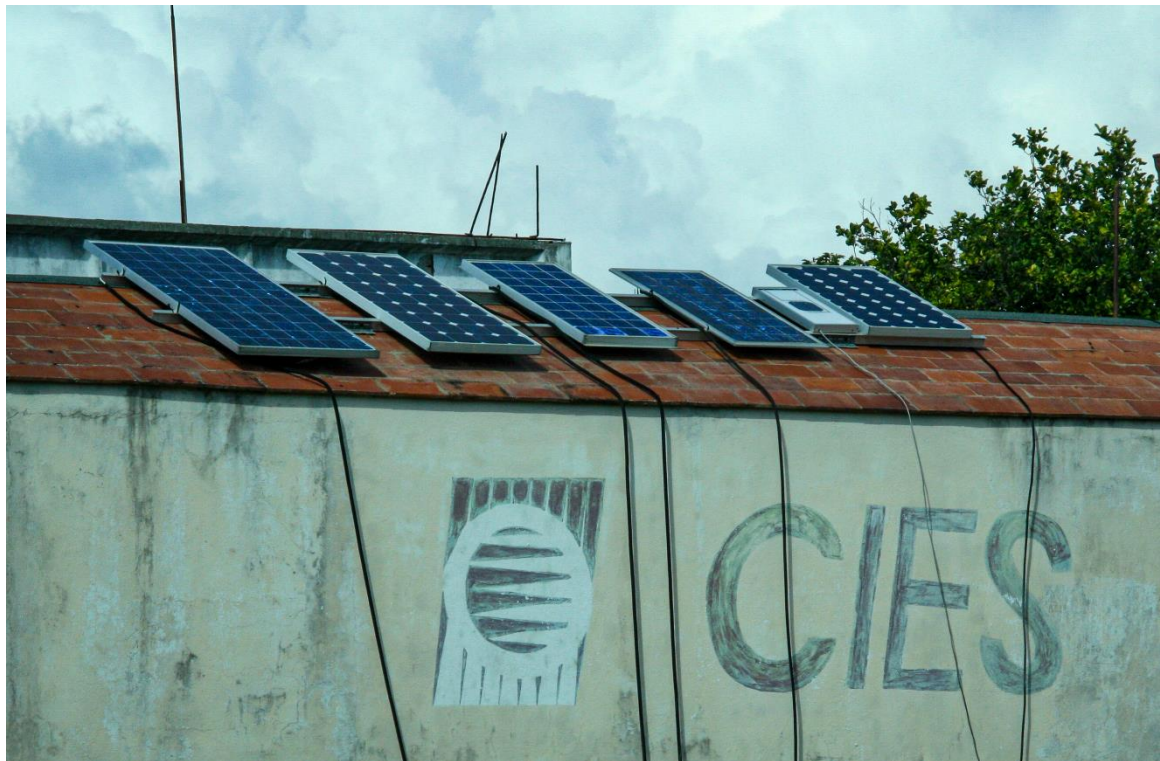
Solar panels, Solar Energy Reseach Centre
