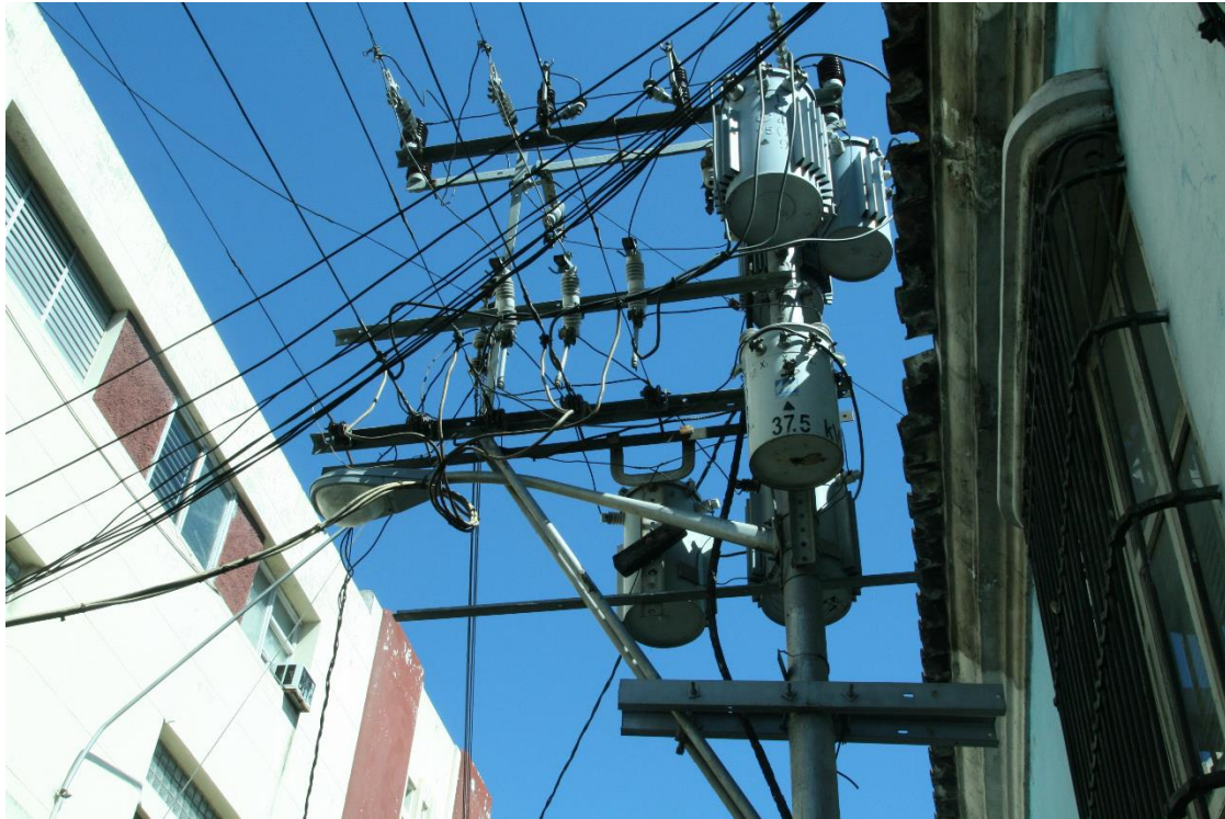
Distribution grid transformers, Santiago de Cuba
