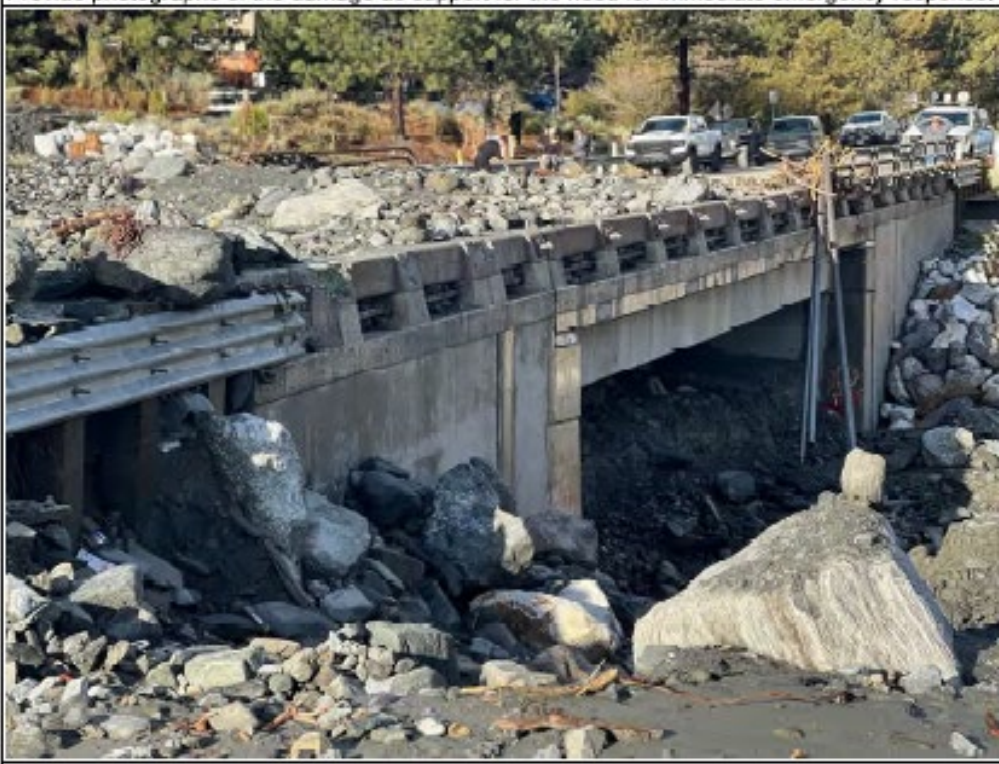
This Photograph Shows: Debris over topped Sheep Creek Bridge (Br No 54 0360), PM 2.44
