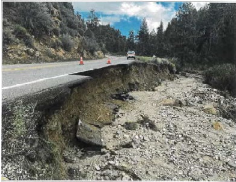
This Photograph Shows: Embankment Erosion and Roadway Collapse at PM 35.47
