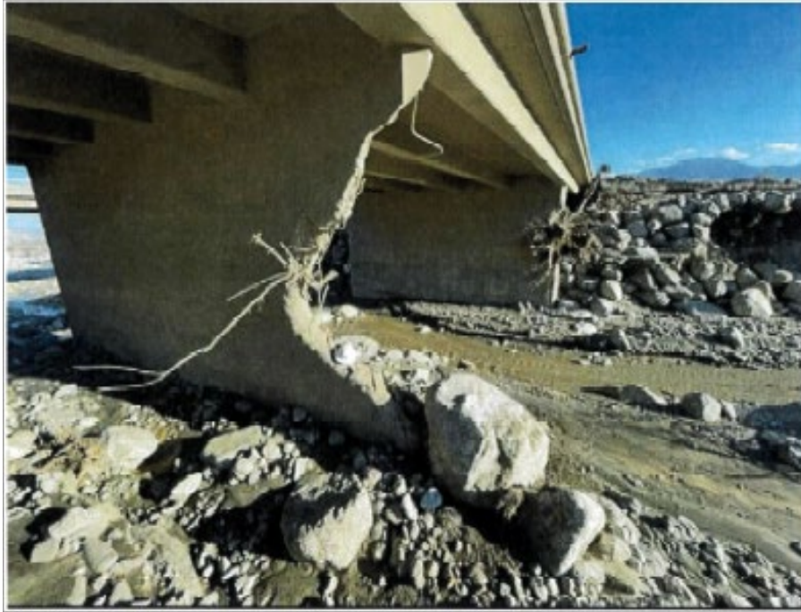
This Photograph Shows: Damaged Mission Creek Bridge on SR62
