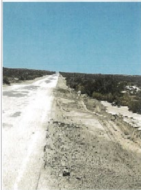
This Photograph Shows: Storm damage on SR62
