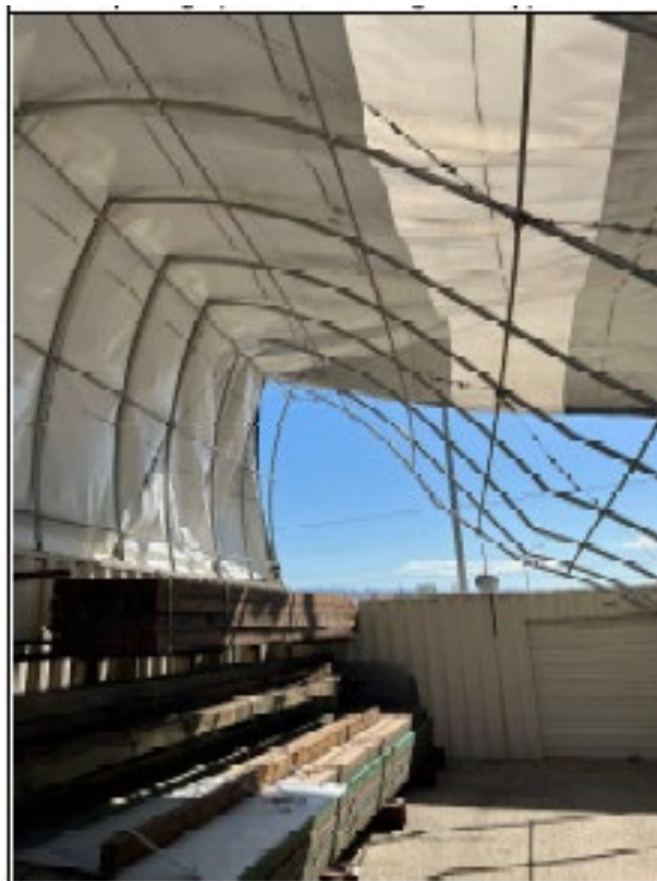
This Photograph Shows: wind damaged canopy
