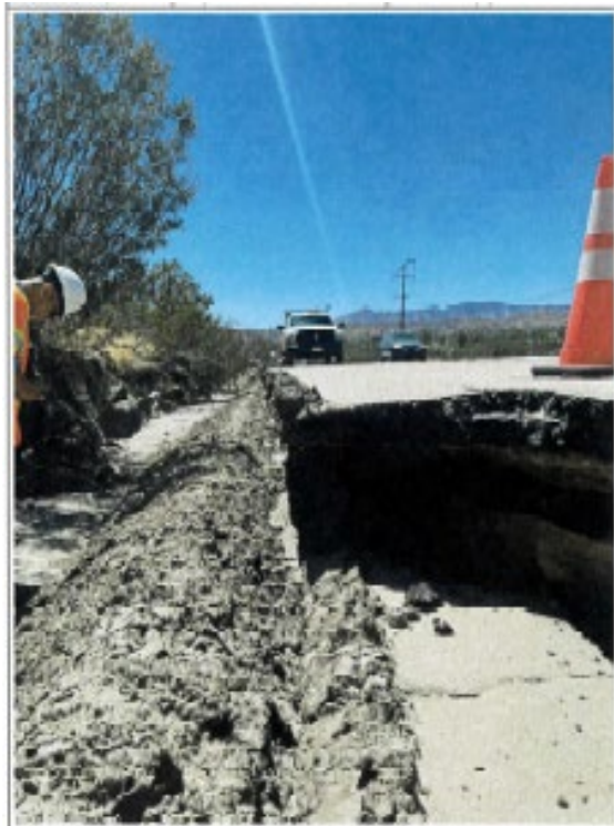
This Photograph Shows: Storm damage on SR62
