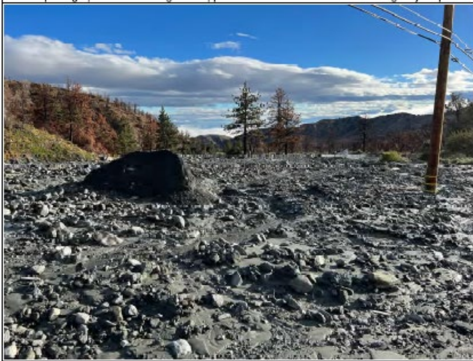
This Photograph Shows: Debris on SR-2
