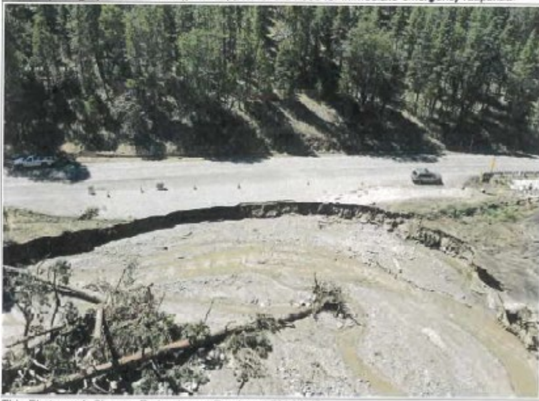
This Photograph Shows: Embankment Erosion at PM 30.40
