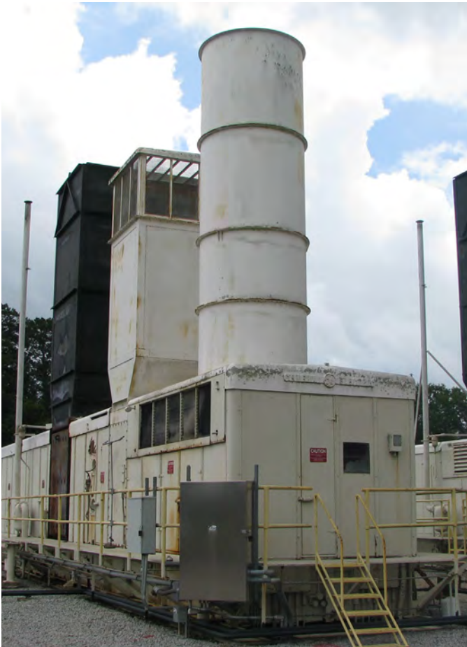
Parr Combustion Turbine
