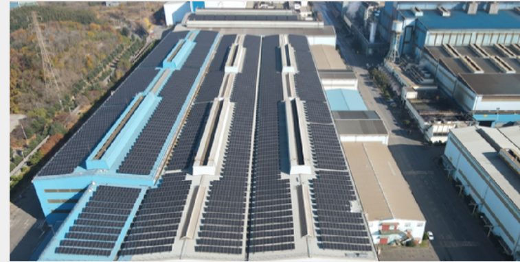
Solar Power Generation Facilities in Pohang Works
