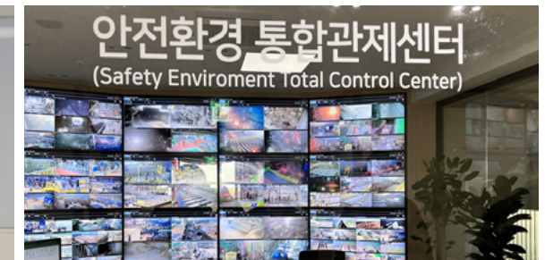
Integrated safety monitoring room
