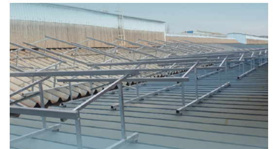
GIX mounting structure for solar power generation used in Pohang Works
