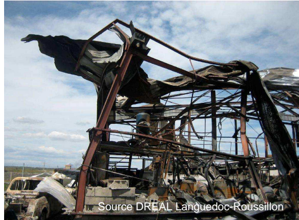
"Flattened" cistern thrown onto a roof
